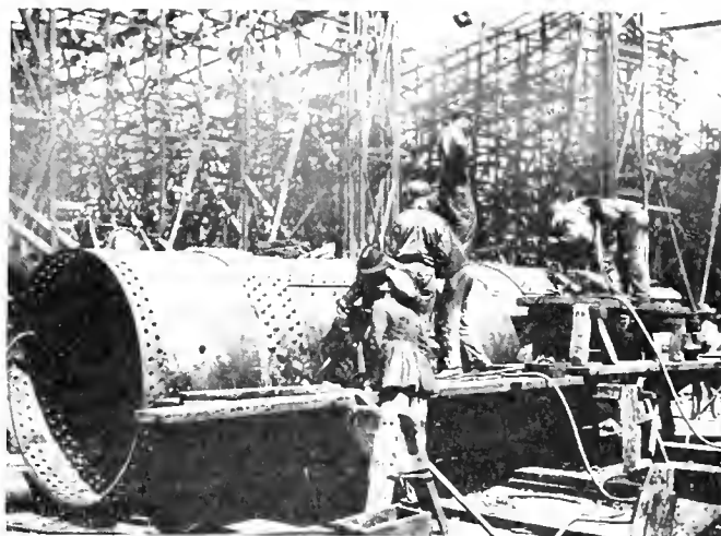
Heavy Pipe Constructed at Plant of Los Angeles Shipbuilding and Drydock Company
