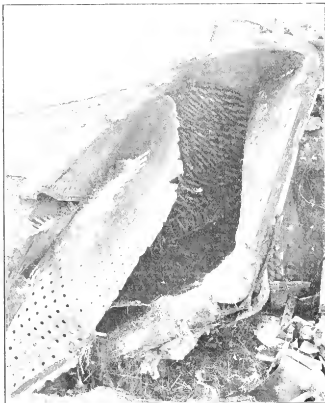
Fig. 3.—Firebox after Explosion, Showing Crown and Flue Sheets Folded Back Against Door Sheet
