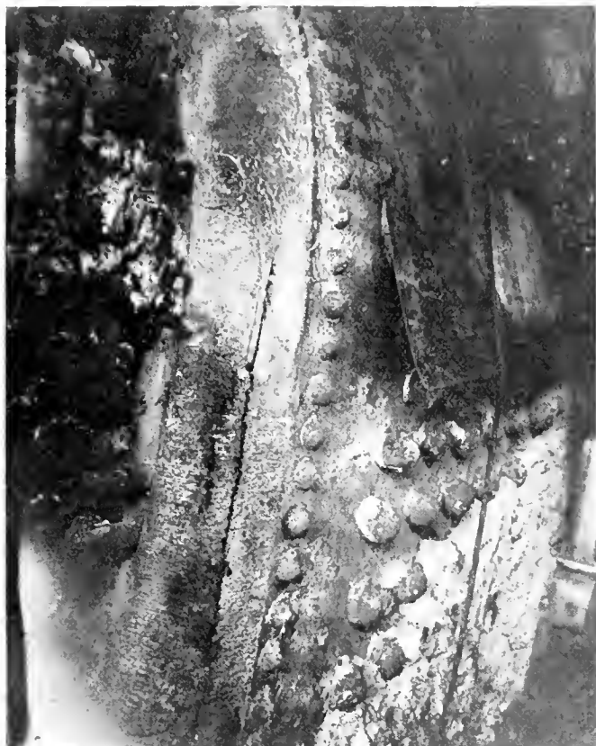
Fig. 3.—Fatal Crack Occurred in a Welded Repair Job
