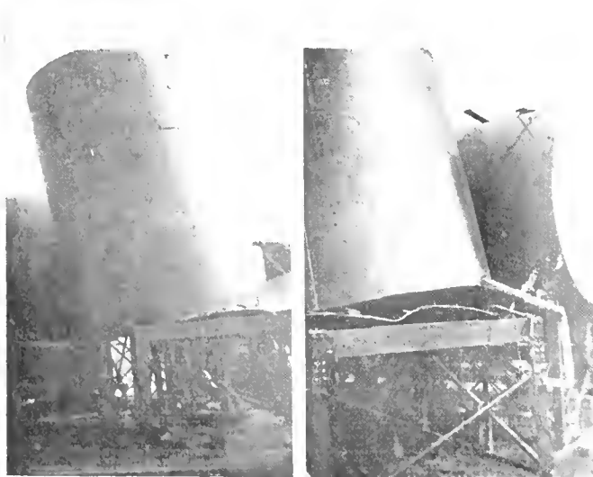
Views of Opening in Bottom Seam of Storage Tank Which Failed
