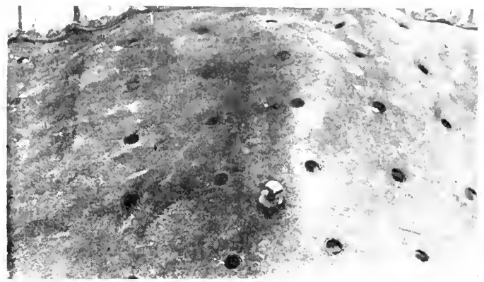
Fig. 3.—Defective Fusible Plug in Crown Sheet Which Contributed to Seriousness of Failure
