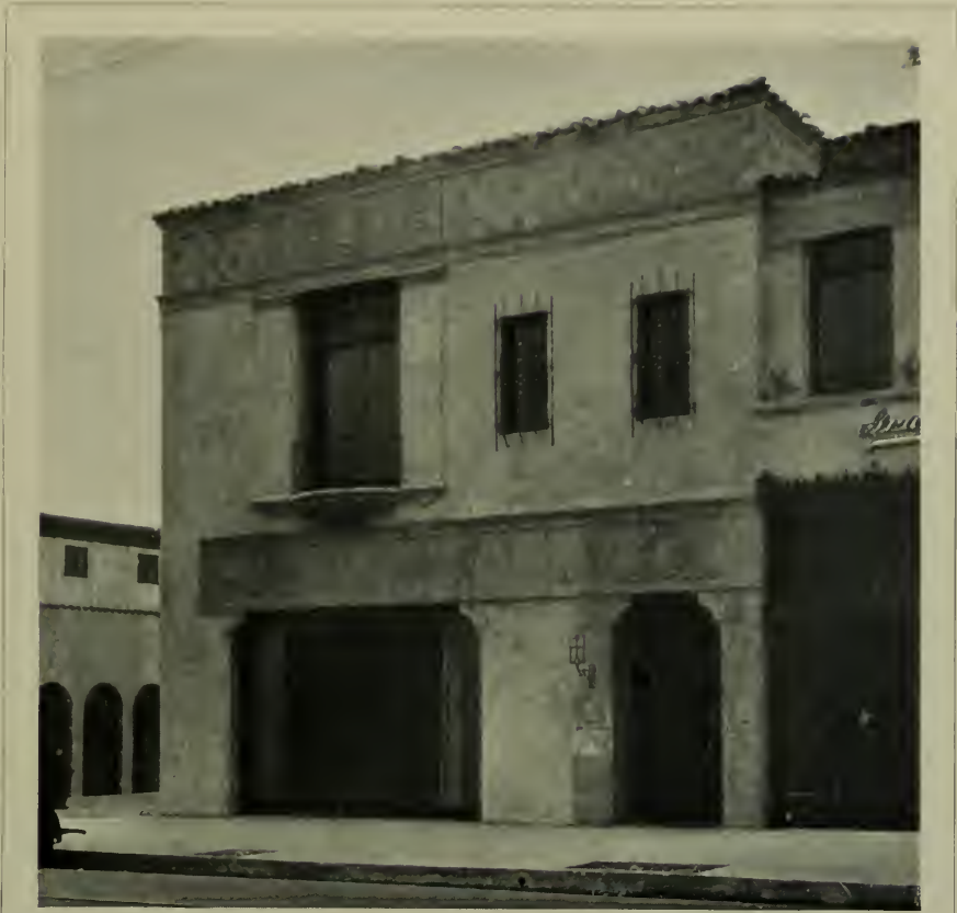
SHOP FRONT DETAIL BILLICHE ESTATE BUILDING, LOS ANGELES. MORGAN, WALLS & CLEMENTS, ARCHITECTS
