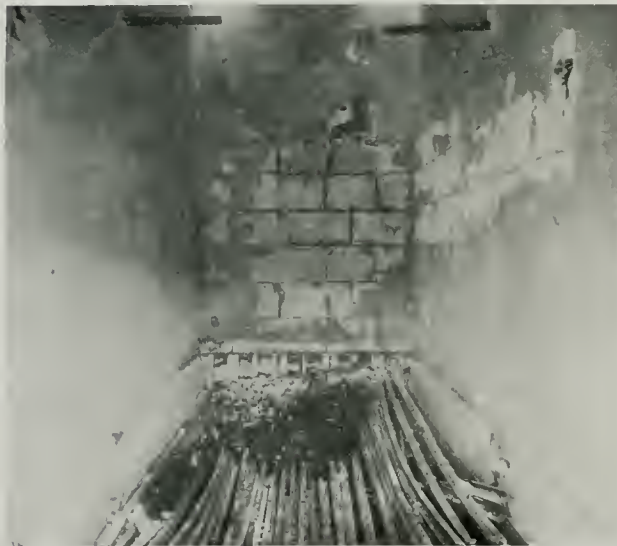
Interior view of building after fire and water
