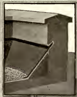
Corner of Roof Showing Concrete Wall with Flashing Form and Flashing Installed
