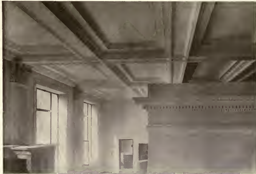
Farmer's Trust Bank, Lebanon, Pa. Richter & Eiler Architects, Reading, Pa. A. J. Lewis, Plaster Contractor.
