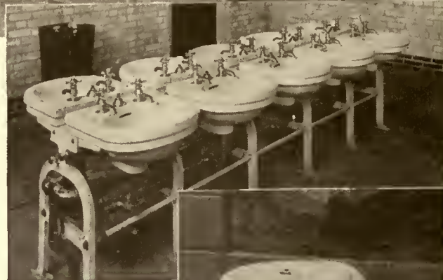
Battery of Crane "Monroe" Vitroware Lavatories with "Securo" Wastes
