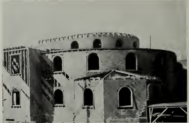
BRICK VENEER CHURCH, SACRAMENTO, IN PROCESS OF DEMOLITION, SHOWING WOOD FRAME IN PERFECT CONDITION
