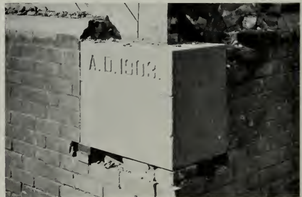
CORNER STONE SHOWS DATE CHURCH WAS ERECTED. WOOD FRAME BACK OF BRICK VENEER IN FINE STATE OF PRESERVATION
