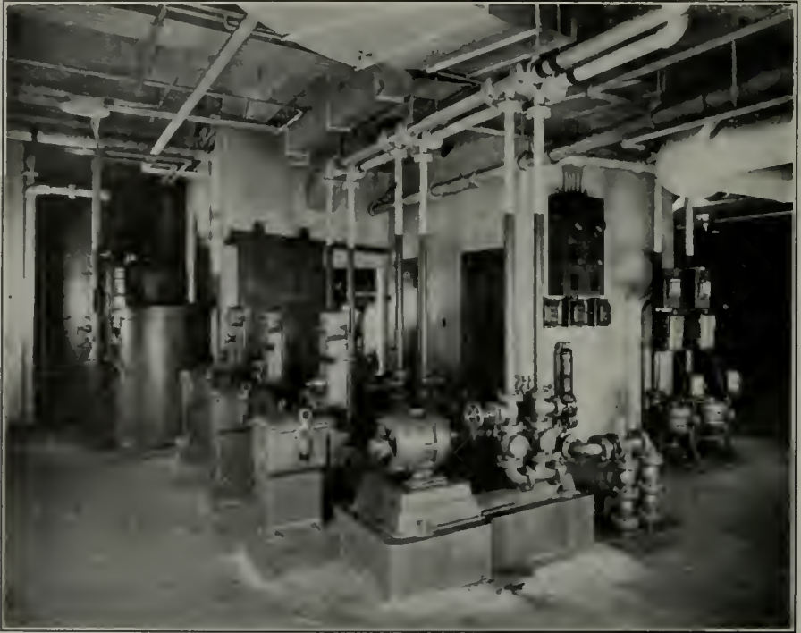
MOTOR EQUIPMENT, MEDICO-DENTAL BUILDING, SAN FRANCISCO Hunter and Hudson, Mechanical Engineers
