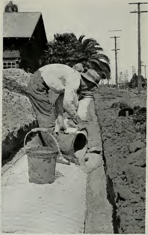
(Fig. 2) SHOWING METHOD OF INSURING A PERFECTLY SOLID BEARING AT THE BASE OF PART CIRCLE ARCHES.
