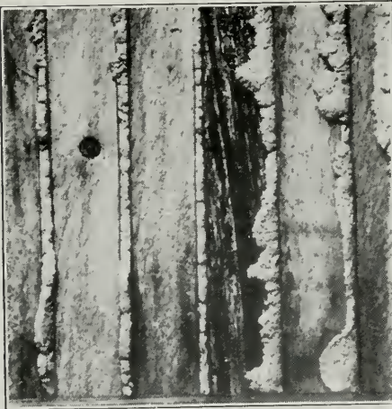
A TYPICAL EXAMPLE OF WOOD LATH CONSTRUCTION. NO PROTECTION AGAINST FIRE
