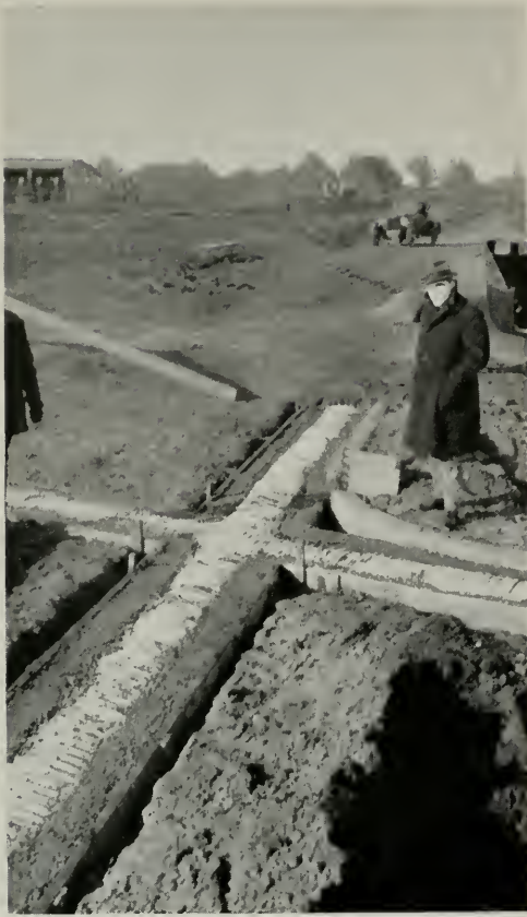
(Fig. 6) PART CIRCLE CULVERT AT INTERSECTION OF CALIFORNIA AND BAKER STREETS, BAKERSFIELD
