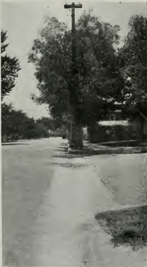
(Fig. 4) SHOWING OLD DIP ON WEST SIDE OF B AND 18TH STREETS, BAKERSFIELD. NOTE RAVELING OF CONCRETE CAUSED BY JOUNCING VEHICLES
