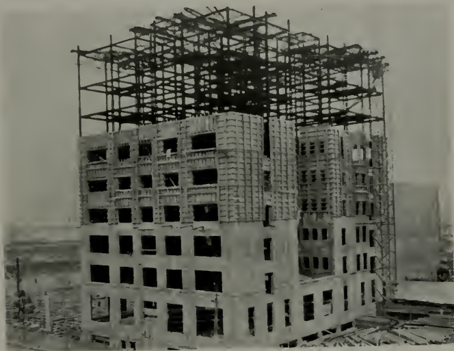
MARUNOUCHI HOTEL, TOKYO Under construction and absolutely undamaged. Steel frame and concrete walls.
