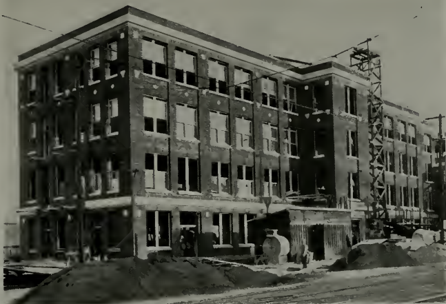
PROGRESS PICTURES, BUILDING FOR THE AMERICAN CAN CO., SAN FRANCISCO Lindgren & Swinnerton, Inc., Builders
