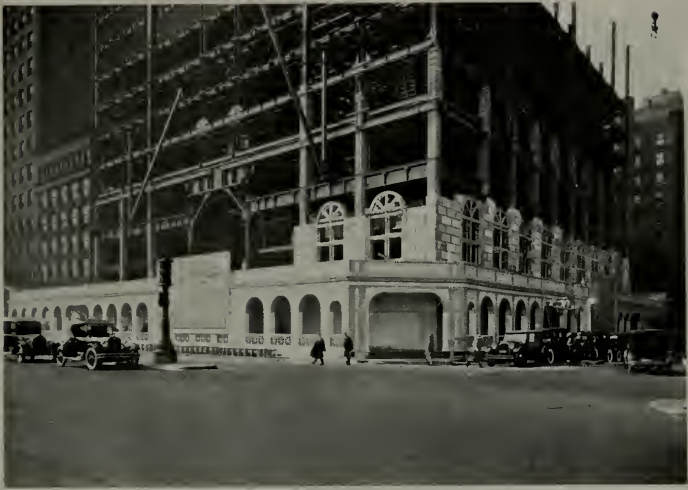
BARRICADE FOR S. W. STRAUS BUILDING, CHICAGO Graham, Anderson, Probst & White, Architects
