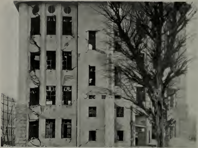
PATENT OFFICE EXHIBITION BUILDING, TOKYO Reinforced concrete. Foundation failure. Side walls settled approximately two feet.
