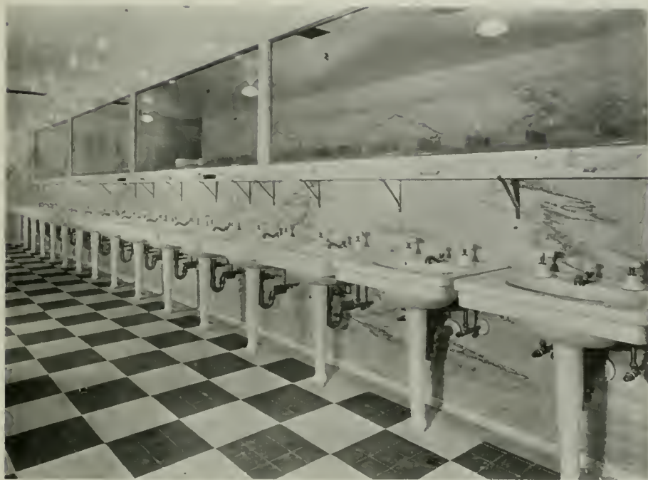
THIS LONG ROW OF LAVATORIES IN THE NEW BILTMORE HOTEL, LOS ANGELES, ARE ALL "PACIFIC"
