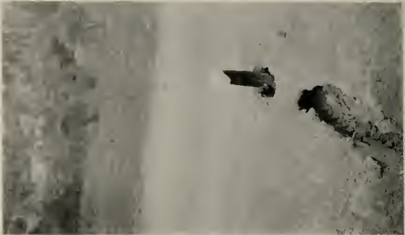
WARNING SIGNAL, PLACED IN HOLE IN THE ROAD CAUSED BY BURNING OUT OF WOODEN CULVERT ON WILDCAT CANYON ROAD,
