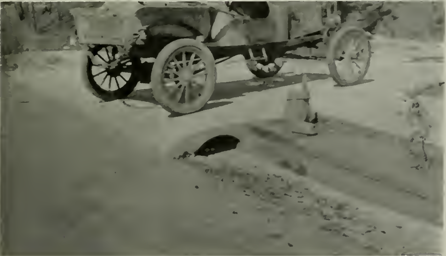
ARMCO PART CIRCLE CULVERTS WHICH HAVE SUCCESSFULLY WITHSTOOD RAVAGES OF FIRE IN BERKELEY'S DEVASTATED AREA.
