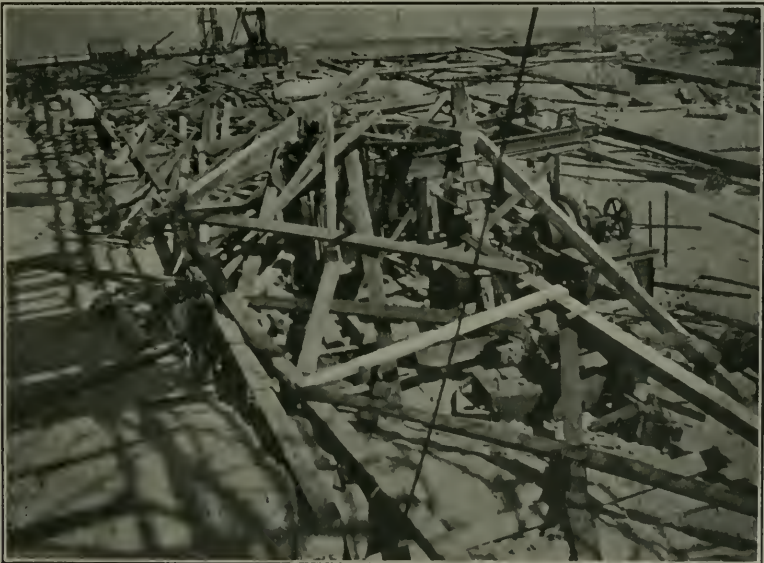
COLLAPSE OF FALSEWORK OF COAL HANDLING BRIDGE, ALAMEDA
