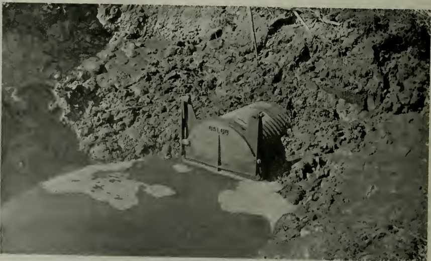
BACK FLOW OF TIDE WATER PREVENTED BY AUTOMATIC DRAINAGE GATE
