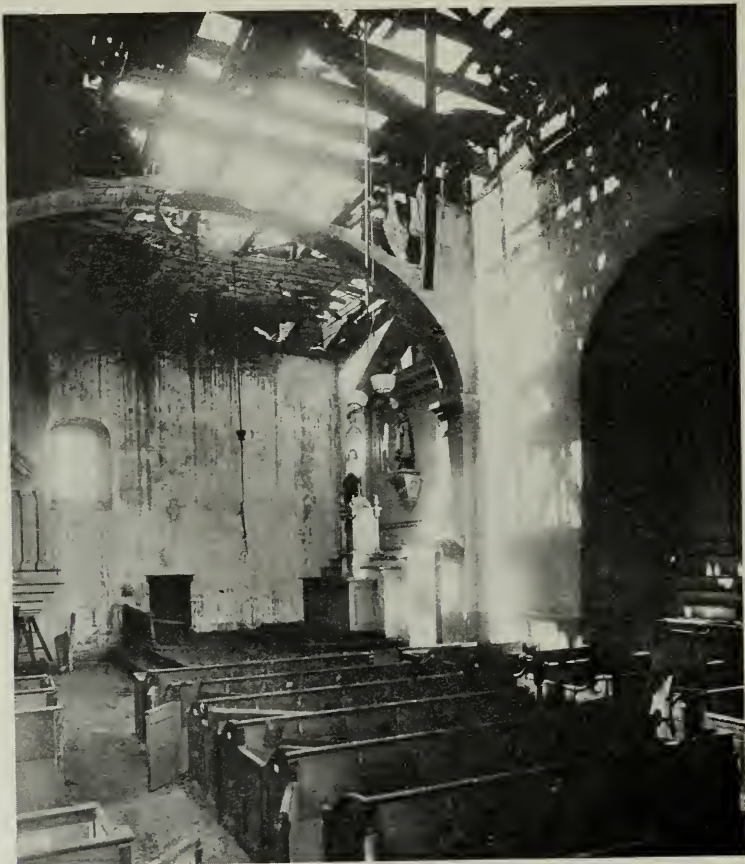
SAN LUIS OBISPO MISSION—THE CHURCH FROM THE ANNEX AFTER THE RECENT FIRE
