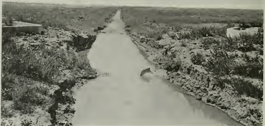
2. Location of corrugated siphon carrying drainage water under irrigation canal. No trouble from expansion and contraction although firmly anchored at both ends.
