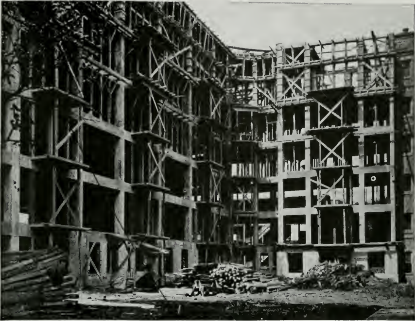
CONSTRUCTION VIEW OF THE BUENA TERRACE APARTMENT HOTEL, CHICAGO Illustrating Some of the Fundamentals Described by Mr. Schlacks
