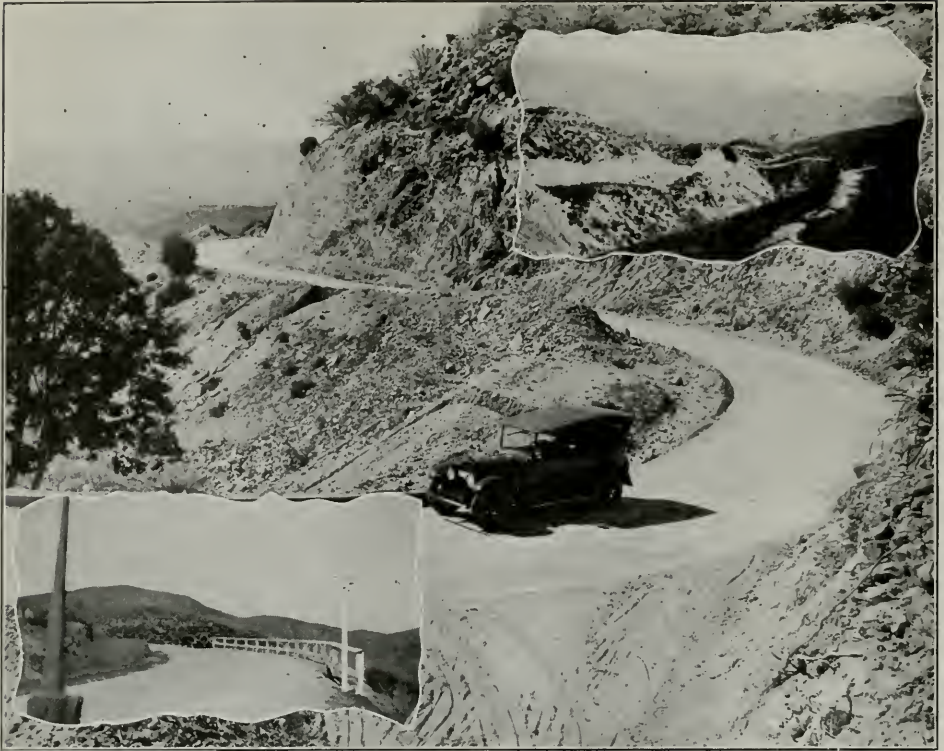
Three Ridge Route Curves. At the Most Dangerous Turns a Curve Such as the Above is "Daylighted" by Still Further Cutting Away of Right-hand Bank
