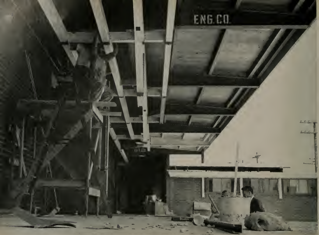
UPPER FOREGROUND shows a section of the 20 x 102 foot overhang. Four by eight foot panels of \frac{3}{4} -inch tongue and grooved fir plywood used effectively to eliminate cost of expensive blocking at unsupported panel edges.
