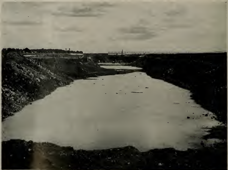
SHIP CHANNEL between Jacques Cartier and Victoria bridges— 3,000,000 cu.yds. of rock excavation in 7,600 ft. of channel.
