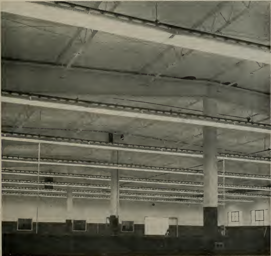
FIG. 1 — LIGHTING FIXTURES in this open-area installation cast an upward light which reduces contrast between ceiling and fixtures and neutralizes any distinct lighting contrast.
