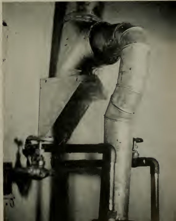
Fig. 1: Typical water heater vent.
