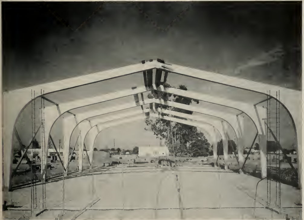
COMPTON-IMPERIAL HOUSING PROJECT—Los Angeles. Side Wall and Roof Framing can be erected in a matter of hours by a small crew with engineered arches.
