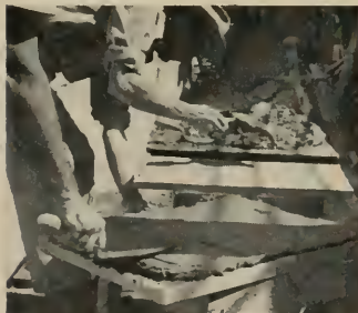
4 Next, slightly more than \frac{3}{8} of an inch of mortar is applied to the C.V. unit. The same amount is also applied to the wall area.
