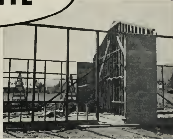
In building this school, BAXCO Chemonited Lumber was used throughout. Treatment standards of the American Wood Preservers' Association were rigidly observed
