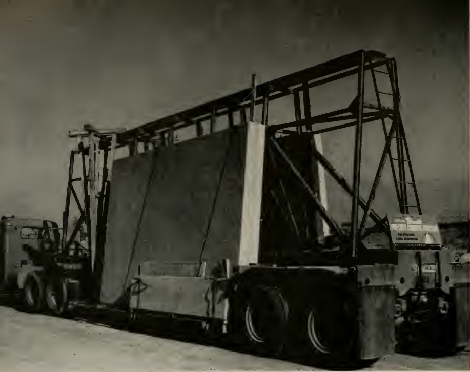
SPECIAL "A" FRAME TRUCKS ARE USED TO TRANSPORT PRECAST PANELS TO JOB SITE. SLABS ARE HANDLED ON THE VERTICAL.
