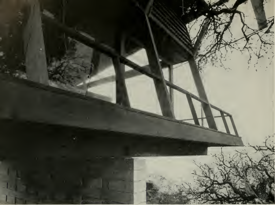
Longitudinal steel girders cantilever well beyond the supporting reinforced concrete block pier to carry floor level out over steeply sloping site.
