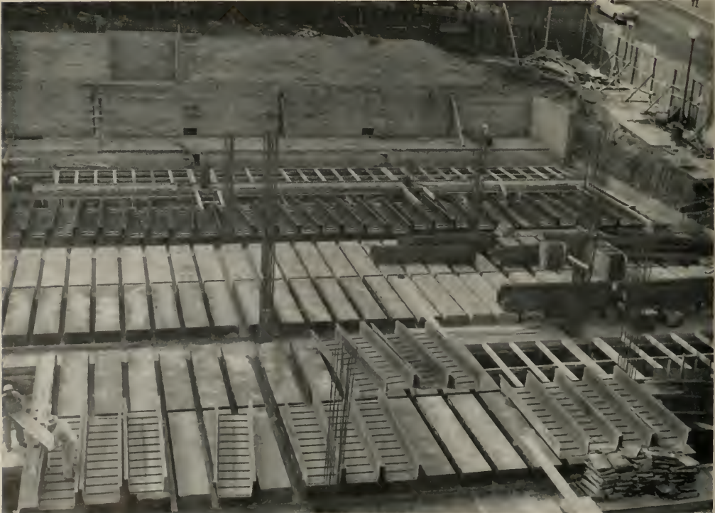
Pan forms in place on the fourth floor near California Street. NOTE how the column bars extend two stories to eliminate any crowding at the splices.
