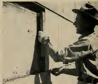
6 It takes the mason only a few seconds to position the C.V. unit and check it with a level. This insures a true wall plane.
