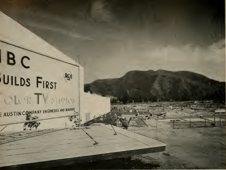
Construction uses a new method for casting and then placing precast concrete wall panel in position.
