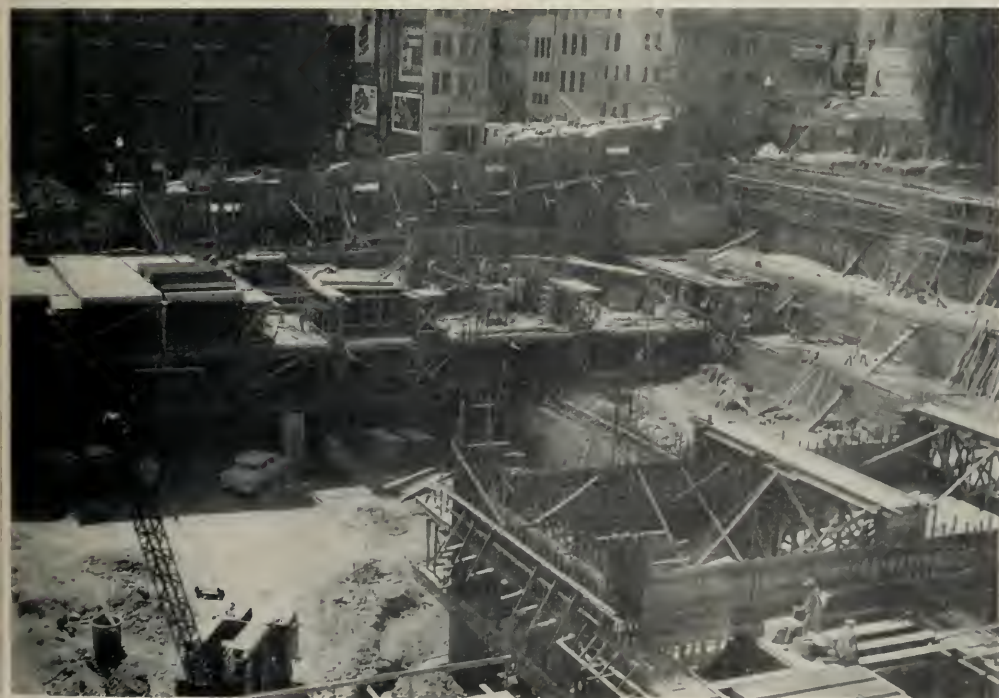
View of the Pine Street section, completed through the third floor, with forms being placed for the fourth floor. NOTE semi-circular ramp, stepped walls.
