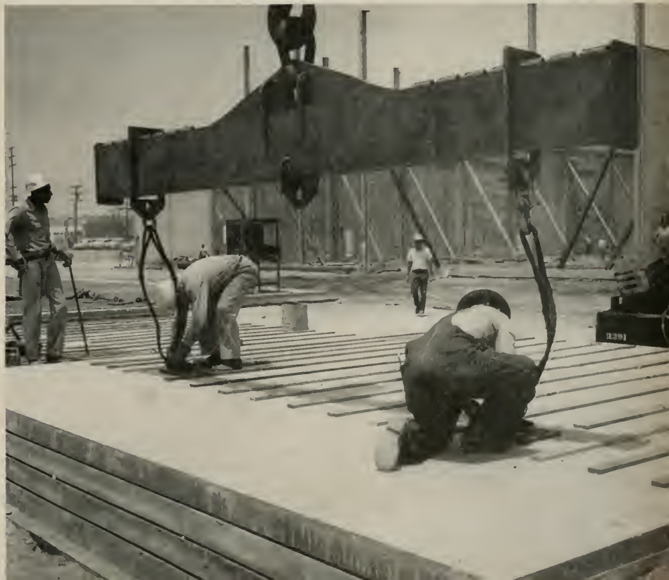
Speedy erection of precast concrete walls—the large lifting plate, raised by a special crane, picks up panels by means of cables fastened to anchorages welded to the reinforcing steel in panels.
