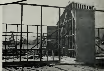
In building this school, BAXCO Chemonited Lumber was used throughout. Treatment standards of the American Wood Preservers' Association were rigidly observed.
