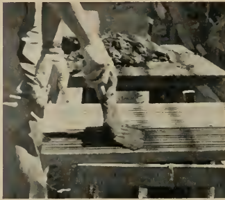
2 Immediately before setting, the back of the Ceramic Veneer unit should receive a brush coat of neat Portland cement and water.
