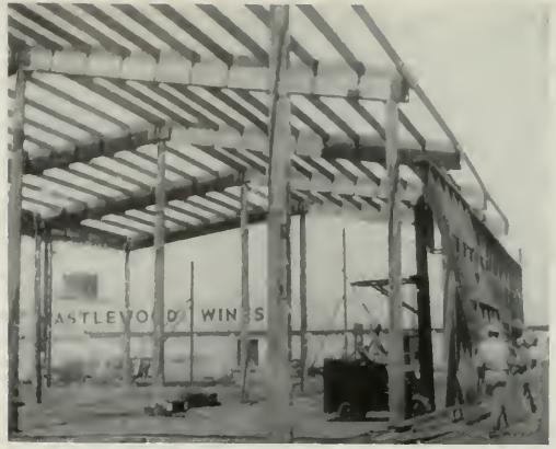
SHOWING erection of prefabricated wall section of United States Products Warehouse in San Jose, California. Walls were raised in 20 ft. sections by fork lift truck.
