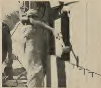
7 He then taps the unit with a rubber mallet to fill all voids, forcing the excess mortar out of joints. Spacers are removed after initial set.
