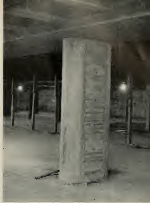
18" x 36" columns from the fourth floor to the fifth floor are smaller to provide wider aisles. NOTE a typical column used elsewhere in the construction is 18" x 54".
