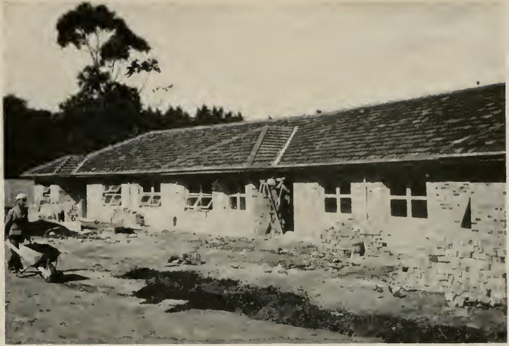
THE CELLS—8'9" by 12'6" and 8'9" by 5", are transported to site and bedded down on standard foundations. Standard brick veneer and marseilles tiles gave this row of units the appearance of a much more expensive construction.
