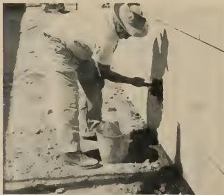
8 Face joints may be raked out and pointed with fine mortar. To complete the job, surface is washed with clean water.
