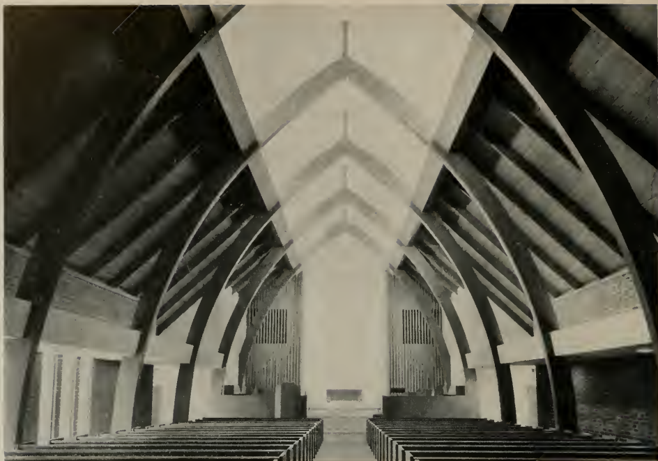
First Presbyterian Church, San Pedro, California. An illusion of floating is given the upper roof section by clever arrangement of free standing Gothic arches and staggered deck sections. Armet & Davis, Architects; F. E. MacDonald, Jr., Engineer.
