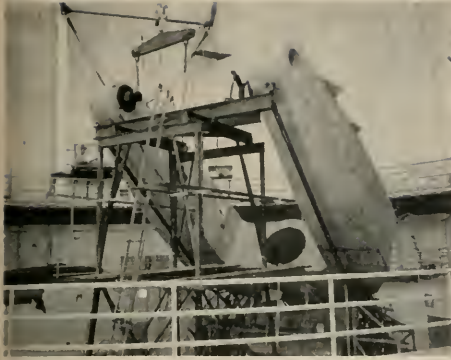
Erection of fork assembly in place supported by the base frame. Scaffolding directly in front of the two fork arms is temporary structure used for erection purposes only. Structure at this point of assembly is approximately 50 feet high.
