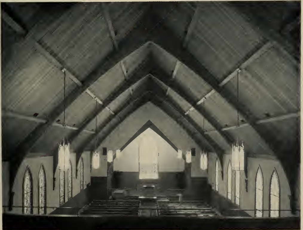
IMMANUEL CHRISTIAN REFORMED CHURCH, Ripon, California. G. N. Hilburn, Architect. Flexibility of modern lamination techniques is illustrated in these arches built up at heel and peak.
