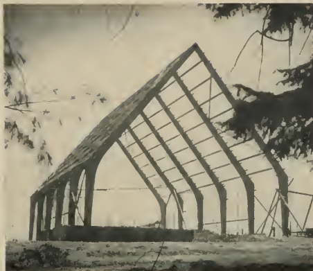
Some idea of the simplicity of erection problems can be had by a look at this skeleton of laminated arches which provide all the structural elements of the St. Albert the Great Church.
