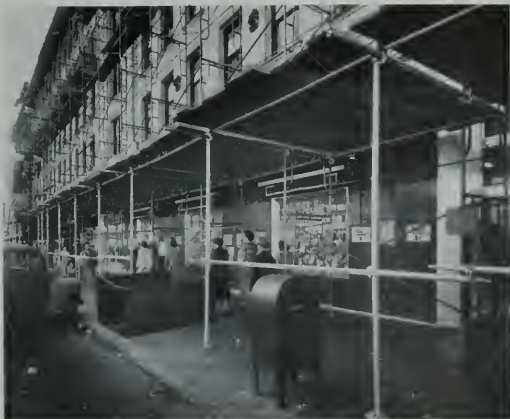
Aluminum and steel type scaffold is used in this instance to provide a safety sidewalk canopy as well as a base for the superstructure on the Shattuck Hotel in Berkeley, California.
