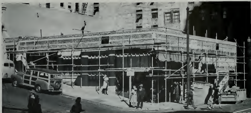
Aluminum scaffold provides level working platforms and minimum sidewalk obstruction for this sloping San Francisco work site Moulin Studio Photos
