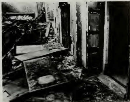
These swinging doors in the Lynn High School were a major factor in saving the balance of the school when the auditorium section burned with a loss estimated at $250,000.
