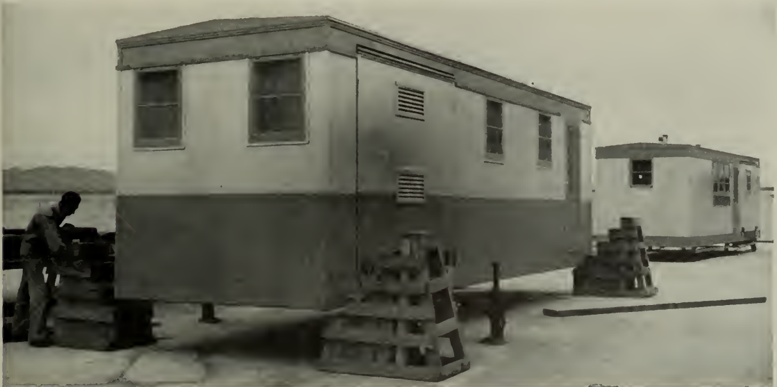
Simple method of loading and unloading a Wingfoot Home with little equipment calls for the use of jacks and house steps. The house is jacked up gradually to a height sufficient to back a trailer beneath it. Note that bedroom bays are collapsed to permit movement on the highway.
