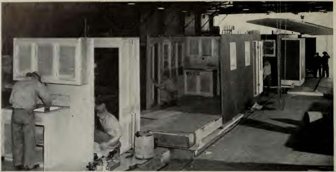
An assembly line view of Wingfoot Homes showing three stages of operation: (left to right), (1) kitchen cabinets and sink being installed adjacent to heating unit; (2) walls of living room being erected and (3) roof being moved into place.
