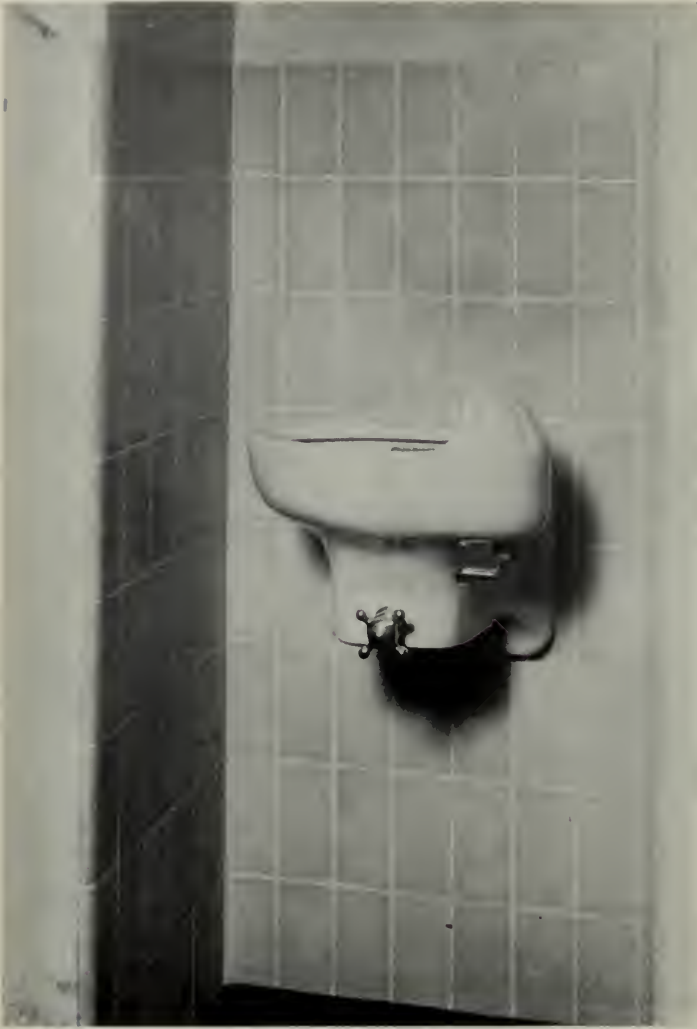
GREEN TILE recessed drinking fountain installation at the new Herrick Hospital, Berkeley, California.
