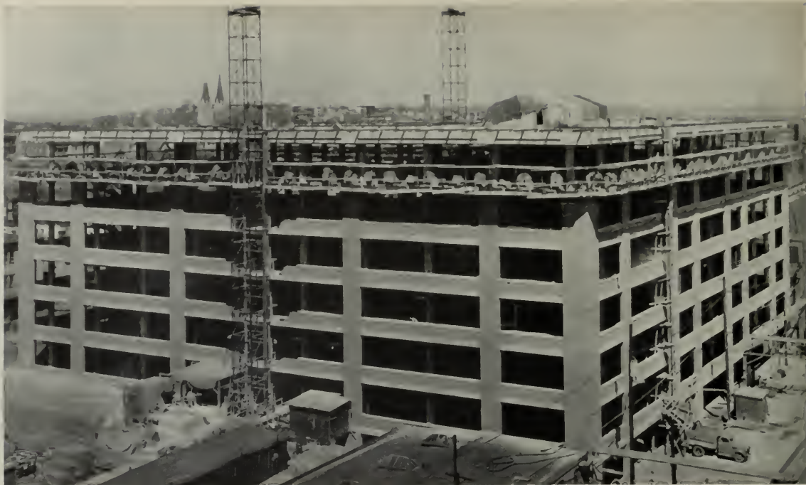
UPPER VIEW is the new six and one-half story building of reinforced concrete and brick construction with an area of 240,000 square feet which is being built by THE STANLEY WORKS, INC. , of New Britain, Conn. It will house machinery for manufacture of regular hardware lines on an expanded scale to meet postwar requirements of the firm.
