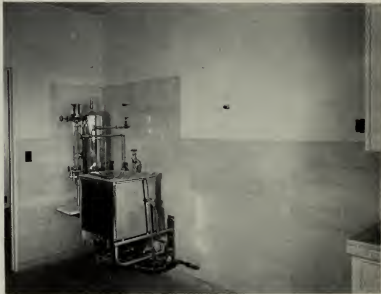
VIEW of portion of Maternity Delivery showing use of oatmeal colored tile on portion of wall for equipment protection.
