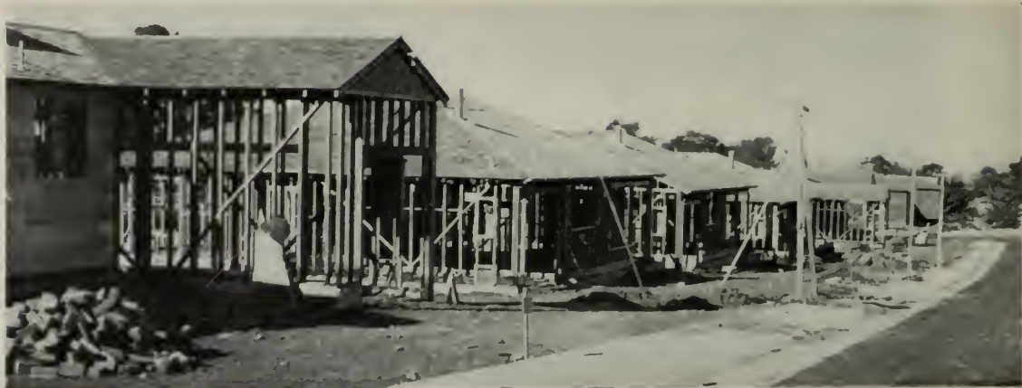
WHOLE BLOCKS of four and five room veteran houses rise in Hillsdale, San Mateo County, California.
