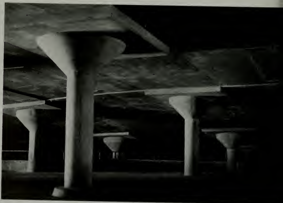
Irregular shaped columns, some 50 in number, serve as floor supports, formed in metal and installed by the Steel Form Contracting Company
