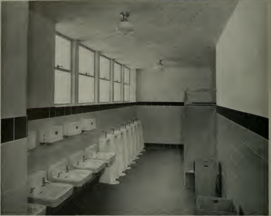
Tile of buff field with brown trimming make an exceptionally suitable color scheme for the boys' toilet room of Ross Grammar School, Marin County, California. The colors are Kraftile's Nevada Buff and Manzanita Brown. The brown bullnose cap extends to the windows' sill. Architect: Carl Gromme; general contractor, Carico & Gautier; tile contractor, Donlon Tile Company. Plumbing fixtures by Crane Company.
