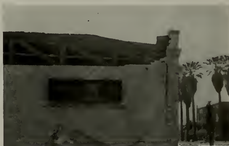
Looking northwest at 618 Linden Ave., Carpinteria, California. Northeast wall tilted out two inches and separated from the southeast wall.
