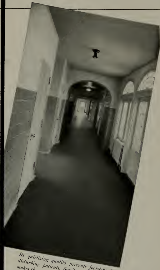
Upstairs and down, corridors in the Home and Hospital for Crippled Children, West Orange, New Jersey are floored with Nairn Linoleum.
