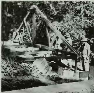
Standard 32-foot span timber roof truss for warehouse at Forest Service Experimental Range Station, Strawberry, Calif. 2 1/2" TECO split ring connectors at all joints.
