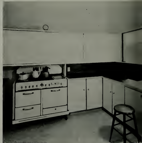
Gas fuel is used for heating, cooking and hot water
