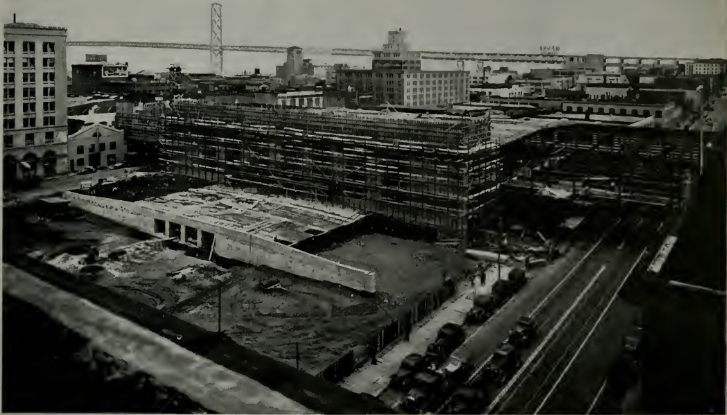
San Francisco Terminal, Facing Mission Street, showing center unit under construction. Street car ramp in the foreground. East and west units not visible.
