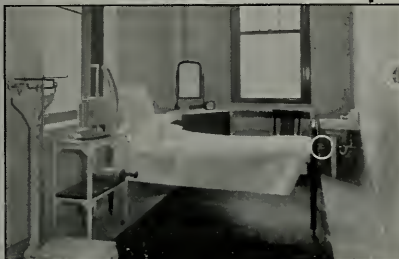
Basal Metabolism Room, St. Elizabeth's Hospital, Chicago, Ill. Showing Johnson room thermostat and radiator valve
