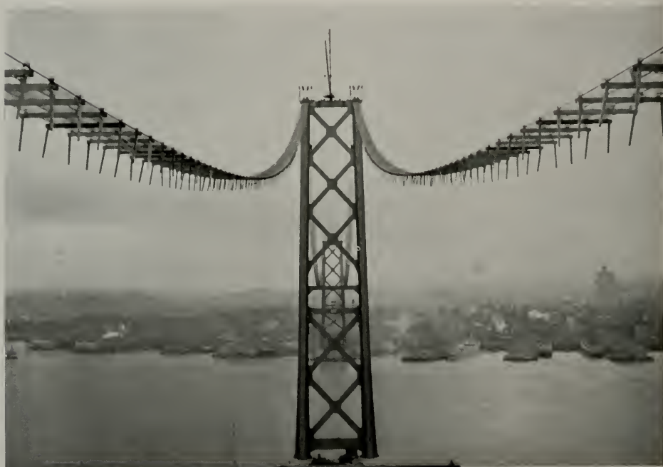
CAT WALKS, EACH TEN FEET WIDE, WITH WIRE MESH FLOOR FOR WORKMEN TO TRAVEL OVER WHILE HUGE CABLES ARE BEING STRUNG
