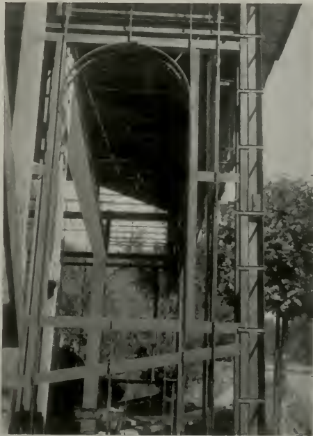
STEEL FRAME HOUSE—Exterior view at south end of garage showing method of using \frac{3}{4} " furring channels around corners and method of using \frac{3}{4} " furring channels for arched window openings.
