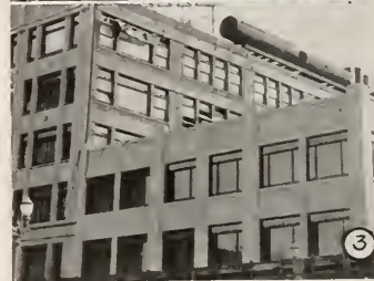
The three views above show a large -core building in which a 3-story wing has been reconstructed with reinforced concrete exterior walls and plaster finish, applied to blend in color and appearance with the exterior facing of the main building. (1) Walls being cast in the forms. (2) Removal of form. (3) Completed exterior.
