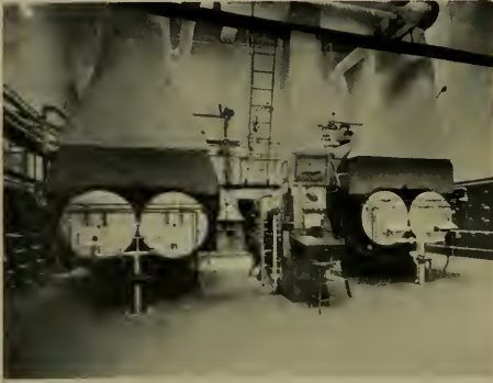
BOILER PLANT, SOUTHERN PACIFIC BUILDING, SAN FRANCISCO
