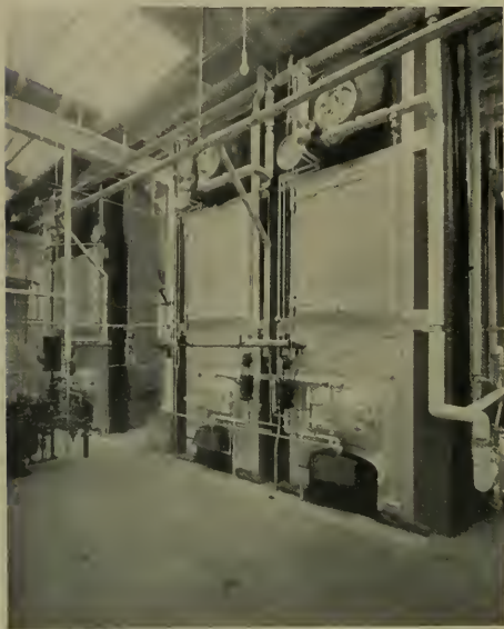
GAS FIRED BOILER PLANT, FERRY BUILDING, SAN FRANCISCO
