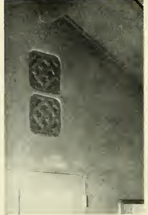
Door in rebate formed in stucco; hinge nails set in stucco. No frame or trim. Chinese tile as heat registers. Ceiling panels fibre board with concrete rafters and girders
