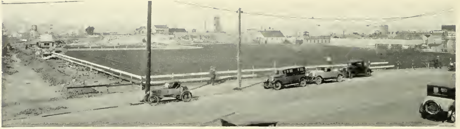
SHOWING GRASS FIELD, SITE OF SEALS' STADIUM Note beginning of form work against rock face in left field.
