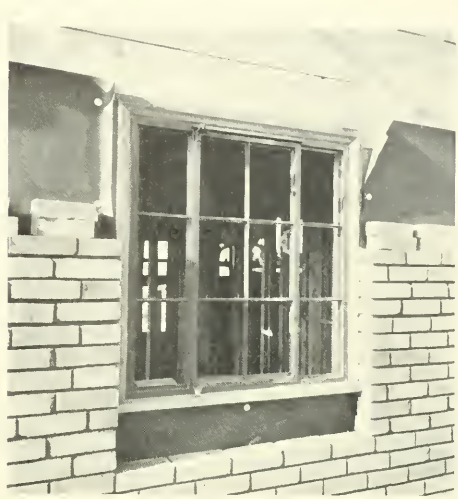
This casement is fitted with "wood surrounds" securely attached with copper-coated screws in a bed of mastic.
