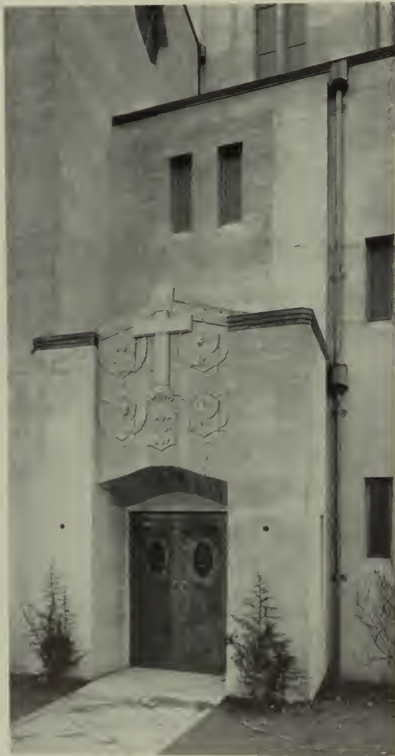
SIDE ENTRANCE, CONCRETE SURFACES, TERRA COTTA LINTEL, COPPER DOORS, ST. JOSEPH'S CHURCH
