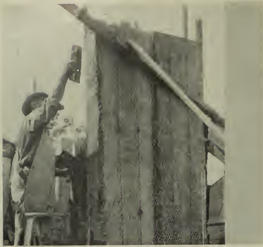
Two channel forms with stucco netting bent around edges at face and reinforced with bars as shown in detail. Edge of channel being buttered with stucco.
