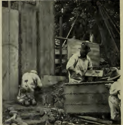
Plasterer in foreground buttering edges of channel preparatory to placing it against buttered edge of preceding channel form.
