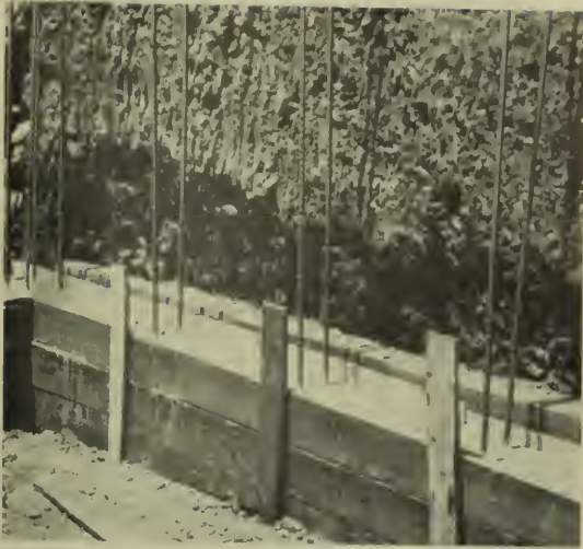
Excavation cut to two inches outside of wall. One-half inch stud bars set at two-foot centers in poured concrete foundation. Hollow tile drain back of wall.
