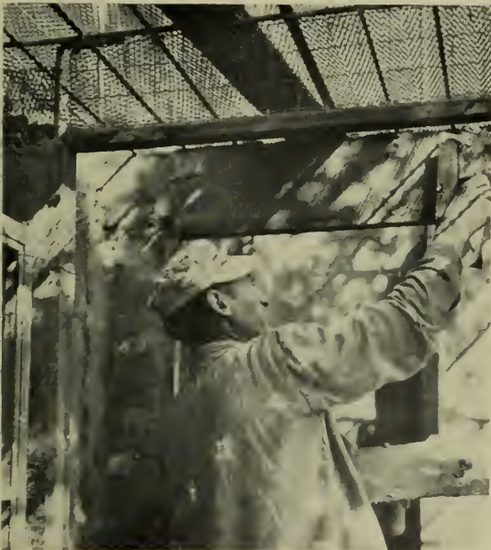
Plastering joists with structural stucco. Plastered both sides within an hour by using a board backing for the side first plastered. Floor slab poured when joists and wall webs have sufficient strength to take load. Joists and under side of slab may be left rough plastered or finish plastered; or ceiling may be wood paneled or finished with fibre board panels sprung between concrete beams.
