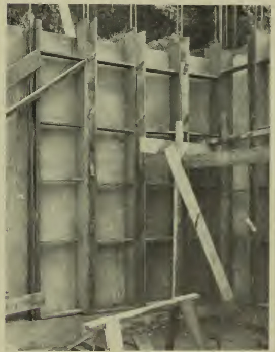
Forms for studs, which were poured; same material as in slabs. Same forms were used on other half of garage.
