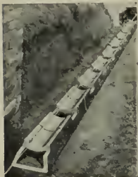
After trench is dug and graded, smooth bottom with sand, stake center line and set Base Drain in place—like laying dominoes.
