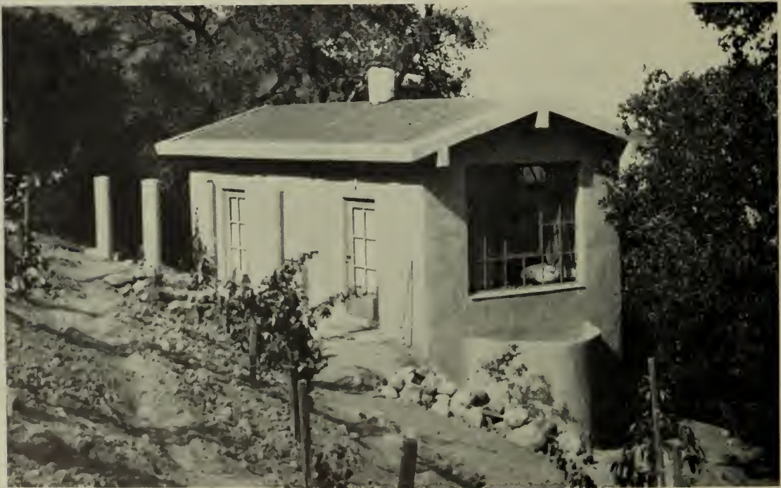
Nearing completion. Tile roof and pergola beams not yet in place. Pergola columns made by bending a cylinder of steel fabric and plastering to one inch thickness. Flower bed wall made by plastering fabric on one side, peeling off paper and then plastering the other side.
