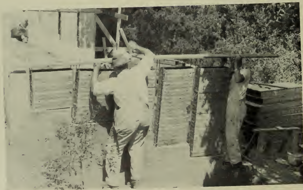
These boxes, stiffened by a zig-zag strip of corrugated board, were then set in position in the wall as shown above, about two and one-half inches between edges of cells. The concrete joist floor and roof systems line with the wall webs, thus forming a series of rigid frames.
