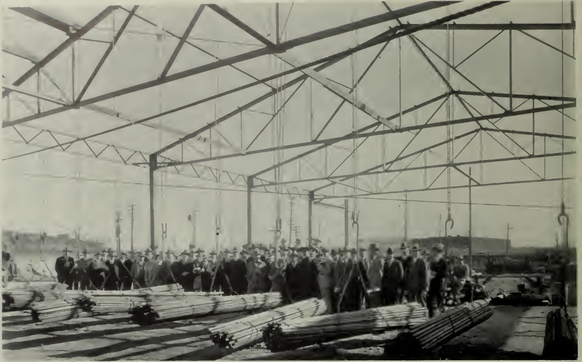
TEST OF ARC WELDED OFFICE BUILDING FOR SOULE STEEL COMPANY, SAN FRANCISCO Five thousand pounds suspended from each panel point in top chord of truss (150 per cent of standard requirements)
