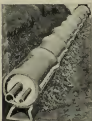
Completed installation of Ric-Wil Type F Conduit. Note Lock Side Joint and ample drainage immediately under Conduit.
