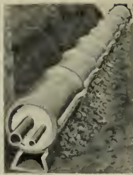
Completed installation of Ric-Wil Type F Conduit. Note Loc-Lip Side Joint and ample drainage immediately under Conduit.
