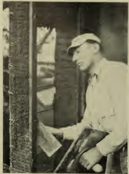
Plastering webs and outer shell of wall with structural stucco wood grounds, split and nailed over web steel prongs, establish exact thickness and depth of web.
