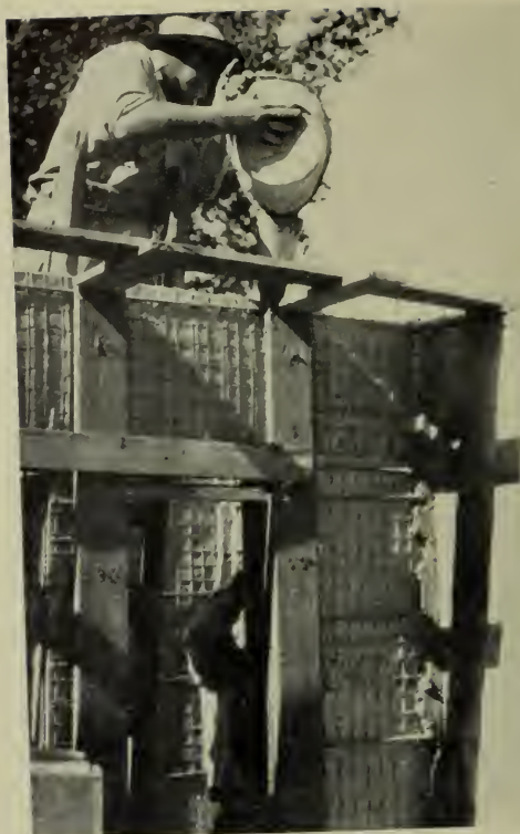
The spaces between edges of cells were covered with wood strips and filled with stucco, thus forming the studs or webs of the wall.
