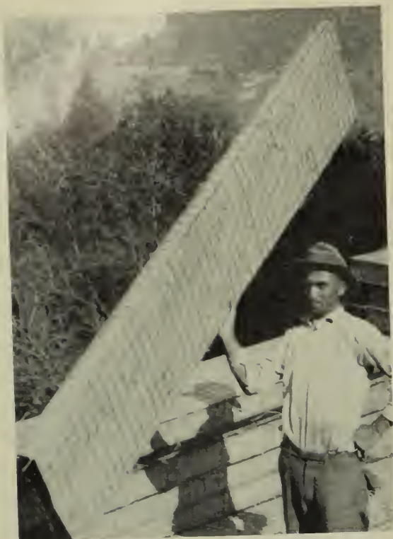
Electrically welded fabric with an attached paper backing was bent in a sheet metal break to the form of long rectangular tubes or boxes, the length of boxes being the wall height.
