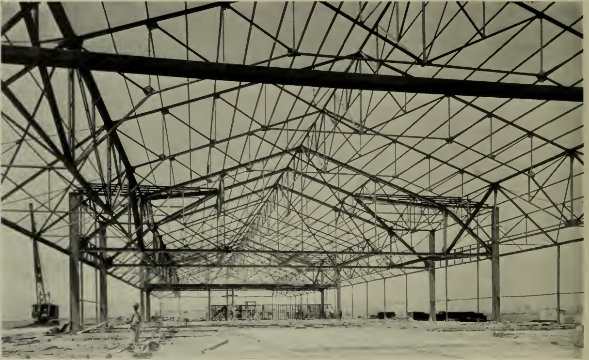
STEEL FRAME OF SAN FRANCISCO BAY AIRDROME HANGAR, ALAMEDA, CALIFORNIA L. H. Nishkian, Structural Engineer
