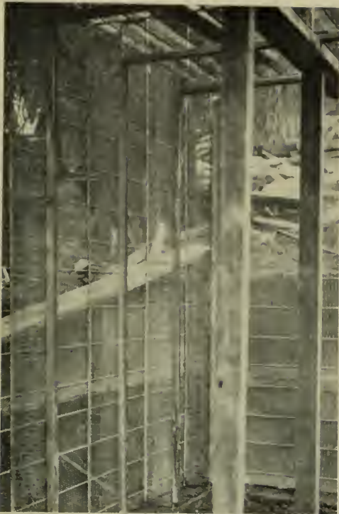
Web reinforcing units with grounds fastened to inner edge were set at proper intervals in foundation. Joist units with grounds on lower edge set in line with webs. Bar lath fastened to outer edges of webs and tops of joists. A brush coat of neat cement is applied as a protective coating and an absorbent of excess water in stucco.
