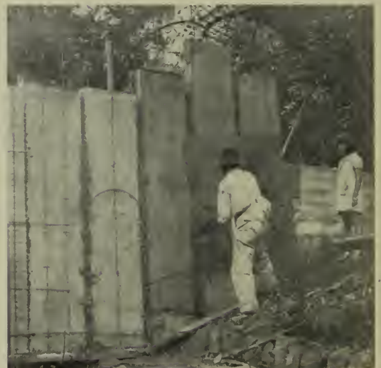
When several studs are formed and before their material has its initial set the outer shell of the wall is plastered on as shown above. Openings are left unplastered and the netting cut afterwards and bent in to form the reveal.
