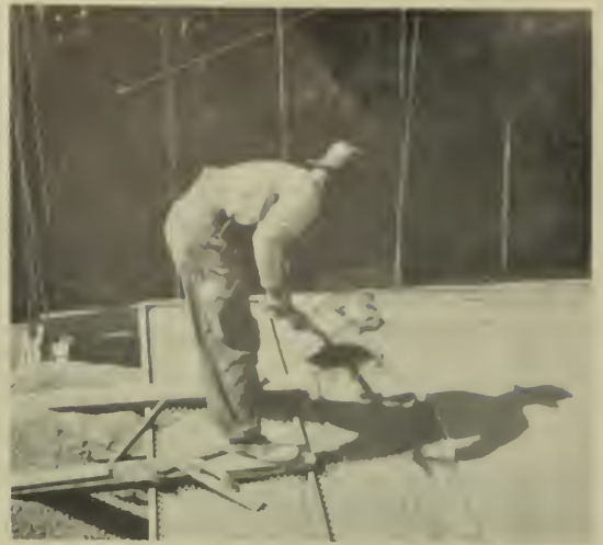
Casting wall slabs on channel forms used in Method D. Slab reinforced with stucco netting bent to form shown in detail drawing on page 89.
