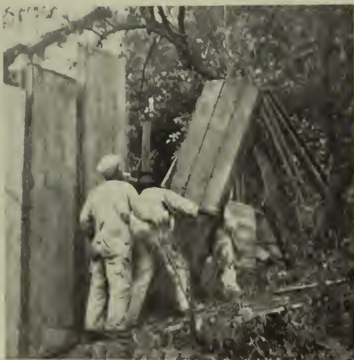
Channel form with buttered edge being placed in position in wall. The two buttered edges are then squeezed together with furniture clamps to form the stud or web.
