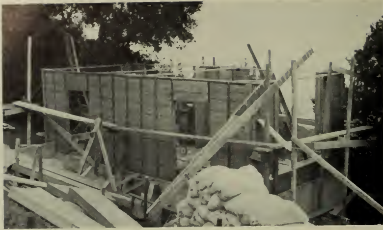
Paper-backed steel fabric boxes in place for main story. After the webs were poured and the strips removed, the wall was completed by plastering the inner and outer faces. Door and window frames were plastered in as the work progressed. In a later development of the same method, the boxes were buttered on the edges and squeezed together as they were put in position to form the webs, thus eliminating pouring.
