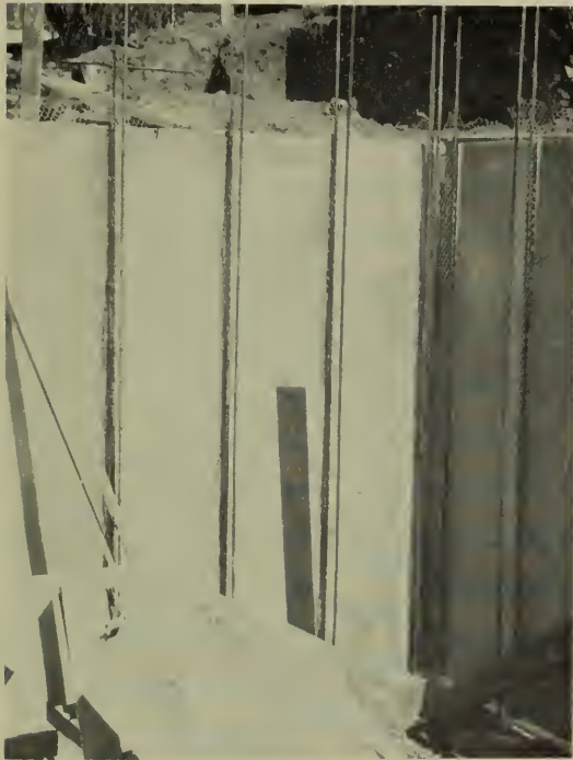
Slabs (cured for one month and waterproofed on back and edges with asbestos fibred asphalt) set on end (by three men) in groove in foundation wall. Projecting netting wired to stud steel.
