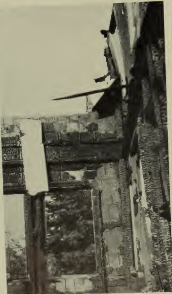
Interior detail of above ruin. Note complete destruction of timber interior and bending of stucco shell at window in upper center of photo.
