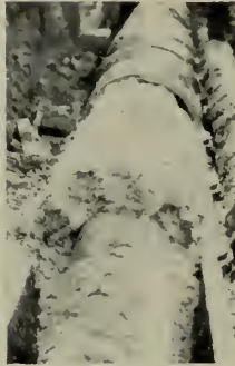
Top conduit section removed to show Dry-paC after installation. An official test of this underground steam heating line showed an efficiency of better than 94%.
