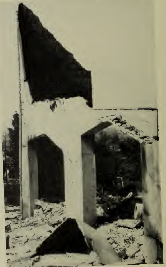
Another proof of the strength of cement stucco. Note fragment in foreground which has fallen from second story.
