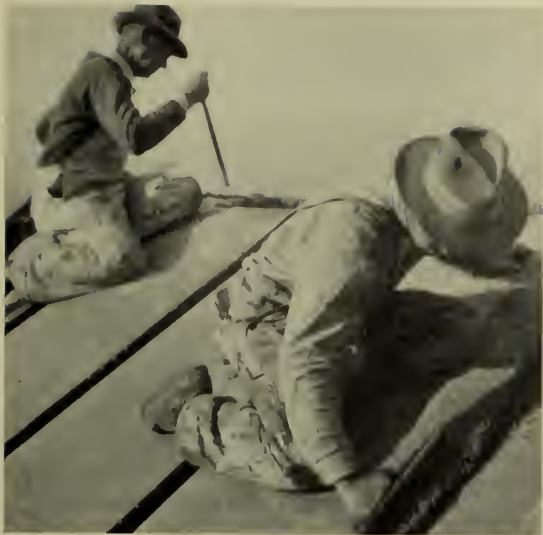
Fibre board boxes, covered on top with case lining paper; rafter steel and ridge girder steel in place. Concrete being pushed and rodded into place in rafters and girder before placing slab netting.
