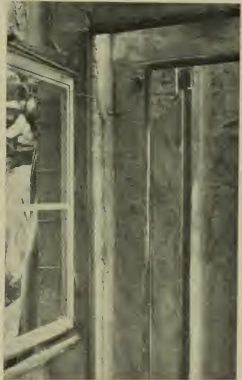
Outer shells, webs and joists plastered. Steel sash and frame set. Bar lath of outer shell cut and bent in to form reinforcing of head and sill. Web grounds may be left to serve as nailing strips for wood or fibre board paneling. Or grounds may be removed and wire prongs used as ties for bar lath for interior plaster or stucco.
