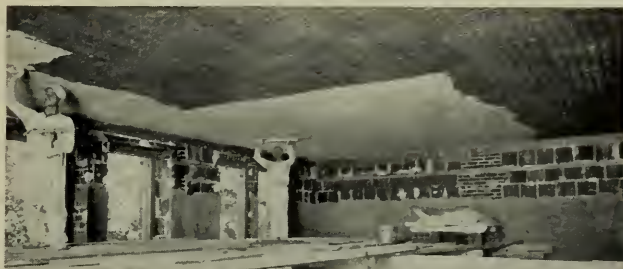
Plastering STEELTEX SUSPENDED CEILING, State Armory, Erie, Pa. Joseph F. Kuntz, Architect, Pittsburgh, Pa. Lee Stearns, Plastering Contractor, Erie, Pa.
