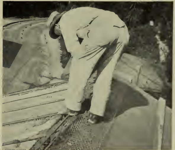
Slab concrete screeded off to one and one-quarter inch thickness. Ridge girder being filled; netting to lap over ridge to form tie.
