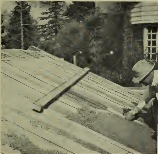
Slab netting in place. Note rods between rafters holding netting to bottom of slab in center of span. Slab concrete being poured.
