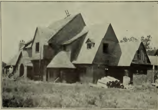
California residence sheathed in Brownskin ready for stucco work Owner, R. T. Creswell. Architect, H. G. McMastern
