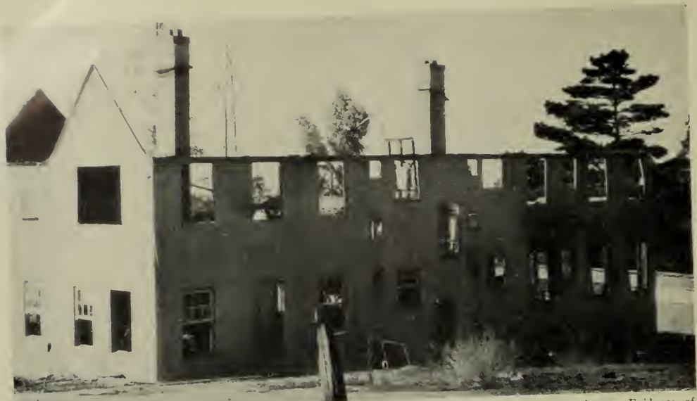
Note one inch stucco shell standing after entire wooden structure which it enclosed had been burned out. Evidence of structural strength in withstanding stresses due to falling floor, roof, fixtures, etc., as well as proof of resistance to fire.
