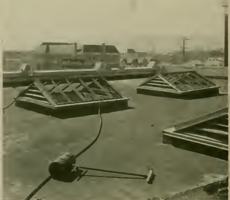
COMPLETION OF MASTIC INSTALLATION. A THREE HUNDRED POUND ROLLER USED TO CONSOLIDATE THE MASTIC
