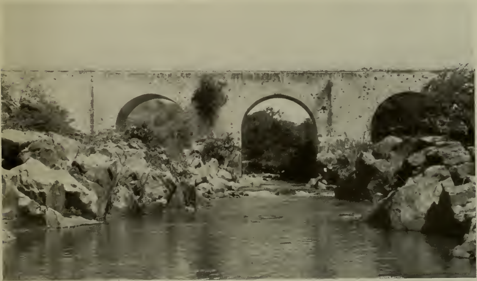
Massive Colonial stone bridge on the historic Borda Stone Highway, between Cuernavaca and Taxco, on the main route from Mexico City to Acapulco. Note shrubbery growing out of the masonry, nourished by heavy seasonal rains. Photograph by the author.
