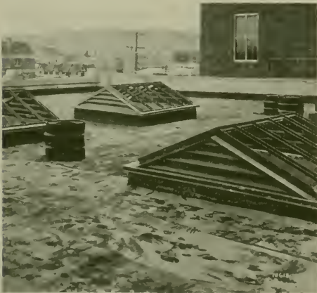
ROOF AREA, SHOWING WIDE MESH BURLAP EMBEDDED IN HEAVY LAYER OF STANDARD PIONEER EMULSIFIED ASPHALT
