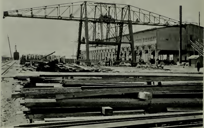
PLATE SHOP, PACIFIC COAST SHIPBUILDING COMPANY, BAY POINT Frederick H. Meyer, Architect
