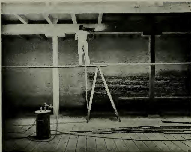
BUILDING FOR ENTERPRISE ELECTRIC COMPANY, SHOWING APPLICATION OF PABCOAT, THE STONE VENEER, TO INTERIOR WALLS
