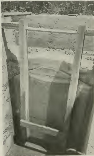
FIG. 1—Automatic Drainage Gate, Ralph Bull ranch, near Arcata, California, on Humboldt Bay. Concrete conduit and wooden cover. Area of conduit approximately 16 square feet. Approximate thickness of concrete 6 inches. The wood gate is not sufficiently sensitive to water level changes.
