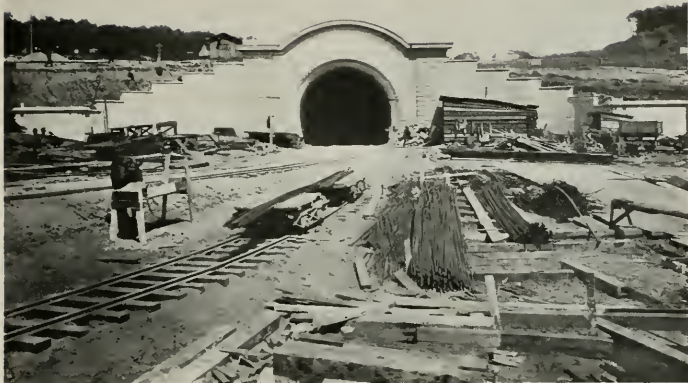
WEST PORTAL, TWIN PEAKS TUNNEL, SAN FRANCISCO. M. M. O'Shaughnessy, City Engineer.
