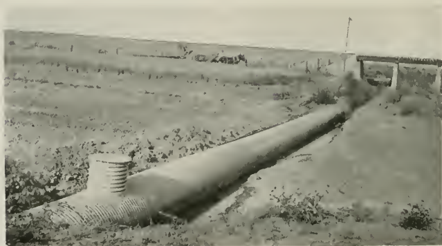
FIG. 9.—Showing 24-inch riser pipe 2 feet high, with bolted top, which is used to clean culvert after flood season.
