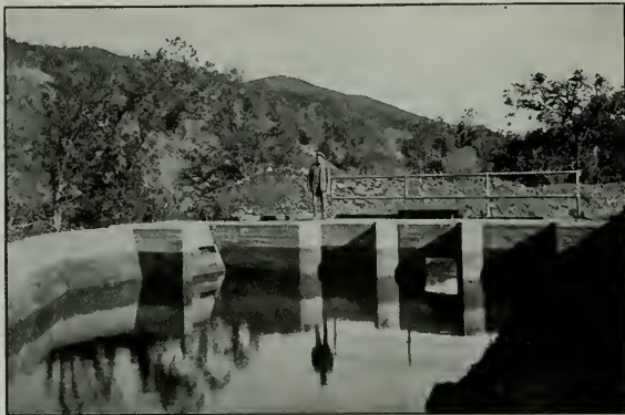
CHECKGATE AT SIPHON SPILLWAY, EAST PARK RESERVOIR, ORLAND PROJECT, U. S. RECLAMATION SERVICE
