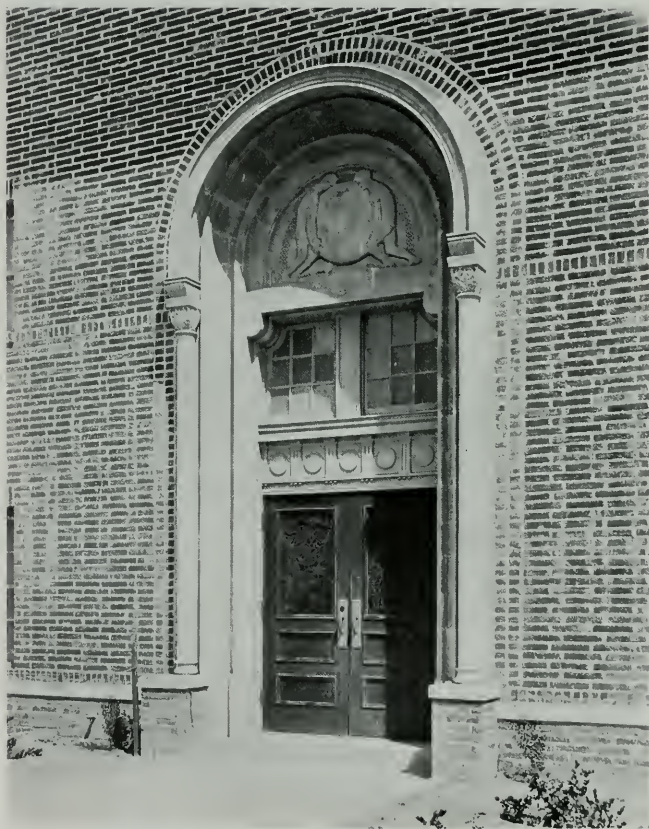
DETAIL, MAIN ENTRANCE GYMNASIUM, LOS ANGELES STATE NORMAL SCHOOL ALLISON & ALLISON, ARCHITECTS W. F. McCURE, STATE ENGINEER
