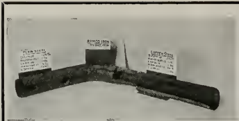
Section of down spout in service under severe conditions for four years. Straight portions of Steel, — elbow of Armco Iron.
