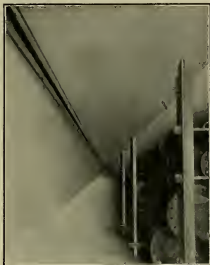
This Tunnel of the Soldier's Home at Washington, D. C., 3000 feet long, 6 feet high, and 5 feet wide,—was made Water Tight by the application of a plaster coat, on the inside of the Tunnel, of Hercules Waterproofing and Strengthening Compound, incorporated with Vulcanite Cement.
