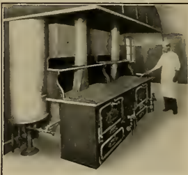
Crude Oil Burners Operating Kitchen Ranges in Government Barracks at Fort Winfield Scott
