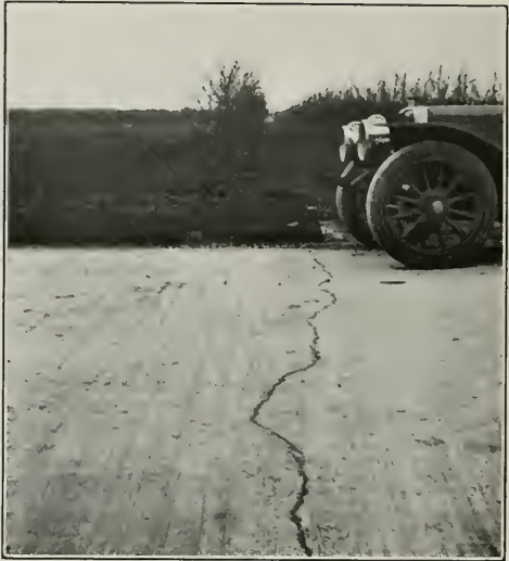
STATE ROAD NEAR SAN JOSE Shrinkage crack
