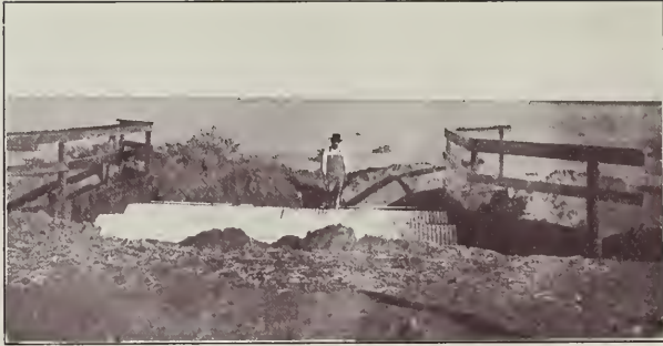
A Pair of Twin American Ingot Iron Culverts, Being Installed in Kern County, Cal.
