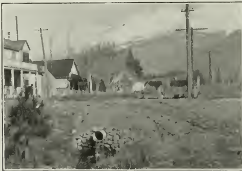
An Ingot Iron Corrugated Culvert Under the Main Street of the Town of Susan. Note the High Snow Capped Peak of Mt. Shasta in the Back Ground
