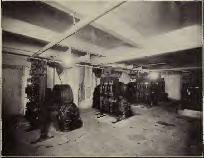
VIEW OF MACHINERY ROOM—PACIFIC ELECTRIC RY. BUILDING, LOS ANGELES SHOWING FOUR CONTROLLER BOARDS
