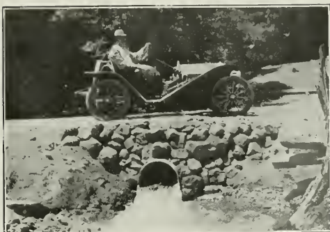
American Ingot Iron Corrugated Culvert under a Placer County Road Between Alta and Emigrant Gap. Installed by Mr. Charles Geisendorfer, Supervisor, the Man in the Automobile
