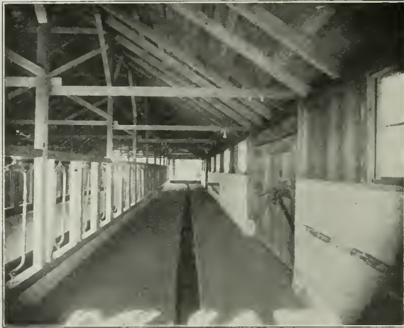
Reinforced Concrete for Farm Buildings—Showing High Foundation Walls and Floor Drainage Arrangement
