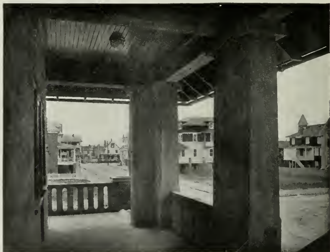
Fig. IV.—View From Front Porch Note strong and massive columns of concrete as compared with light timber construction of houses in the background
