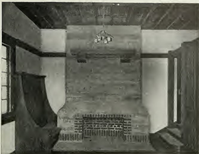
Fig. V.—Living Room Fireplace of Reinforced Concrete. The surface was left as it appeared when forms were removed
