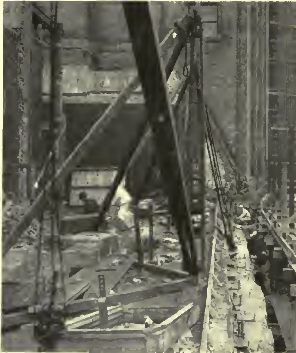
Tenth floor level ready for new walls. Note bolts set in old walls to serve as ties. Walls above this level are of tile faced with stone
