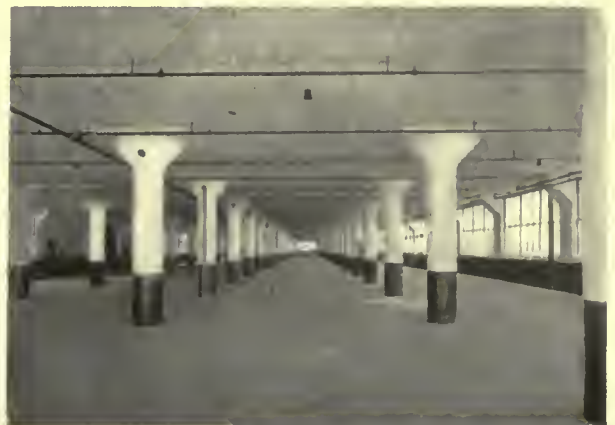
Reinforced concrete. Girderless floor carried on drop-heads. Columns and capitals are round in order to offer maximum resistance to fire.
