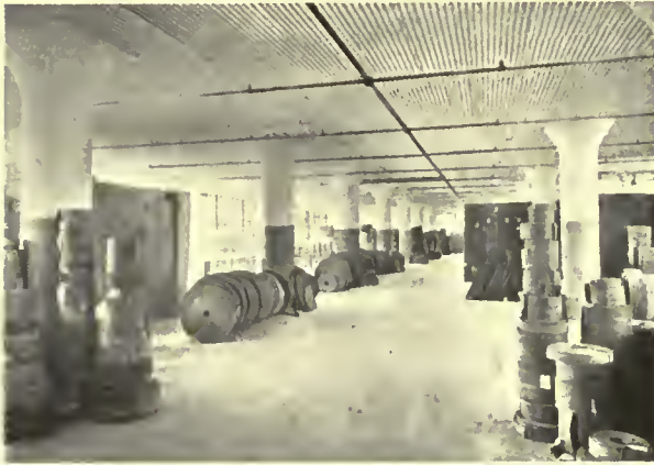
Reinforced concrete. Girderless floor on drop-heads. Corrugated iron used in forms to give ornamental ceiling.
