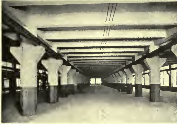
Reinforced concrete. Deep, narrow beams and girders. Heavy cantilevered columns for traveling crane. Wires go through lower half of beams.
