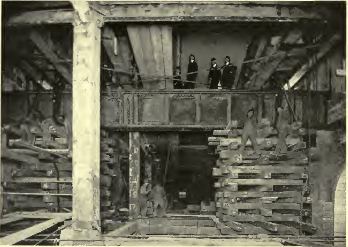
Placing the heavy girders and following with cribbing to minimize damage in case of accidental drop
