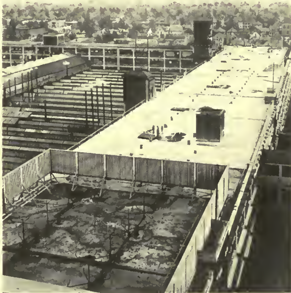
GENERAL VIEW OF COMPLETED ROOF SLABS. SLAB IN FOREGROUND IS ON ONE OF THE BAYS FIRST TREATED, SHOWING FENCES AND SPRAY PIPING IN PLACE
