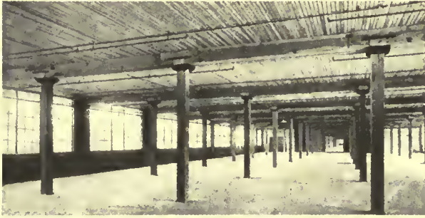
Timber. Mill construction with long span laminated floors. Two piece girders resting on metal post caps.
