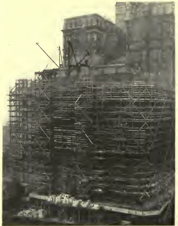
Remodeling No. 1 Broadway 1919-21. Upper stories torn down. Staging in place for the setting of the new stone facing
