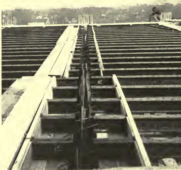
Arctic Ice Cream Co., Detroit, Mich. Steel joist floors framing into reinforced concrete girder of T section
