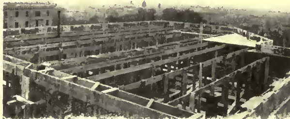
The simplicity of the wooden supports for metal centers is one of the cost reducing elements
