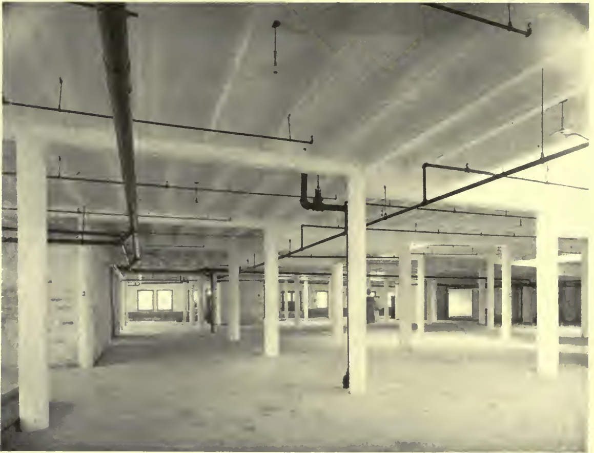
Webb Terminal Warehouse, Philadelphia, Pa., Wm. H. Gravel, Engineer. Unplastered ceilings, ribbed slab floors
