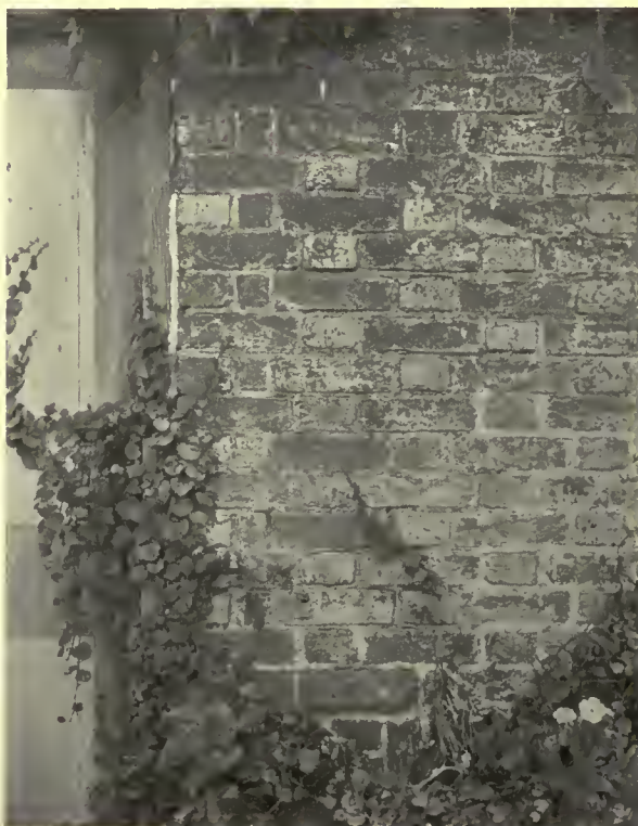
Brickwork, Denn House (1725) on Alloway Creek, near Salem. Some of the stretchers are nearly ten inches long
