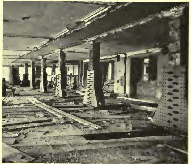
Steel plate bases bolted to cast iron columns to carry loads to plate girders on floor below. Girders are in pairs passing the columns below which were later removed
