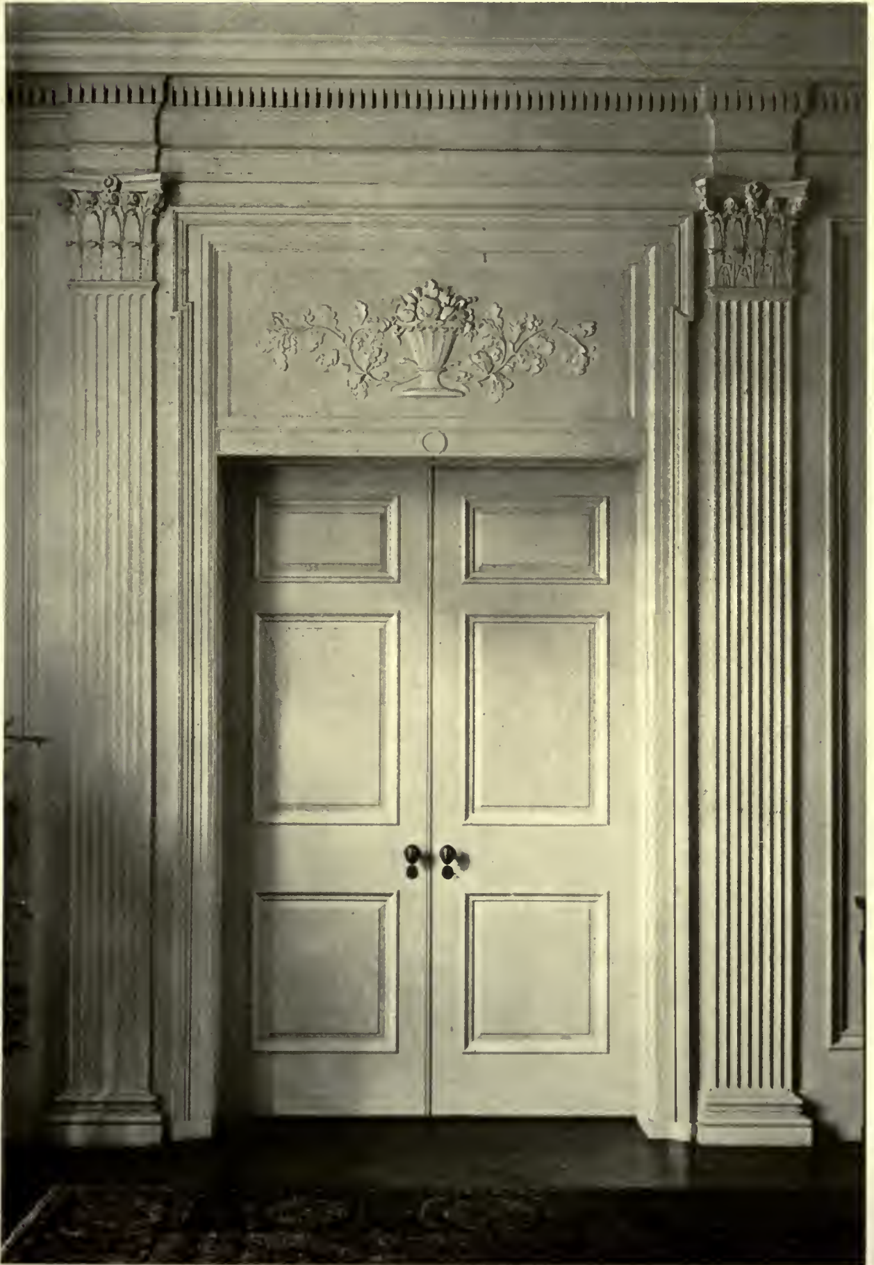
DETAIL OF DOOR IN HALL HOUSE OF LELAND H. ROSS, MADISON, N. J. BEHR & SMITH, ARCHITECTS
