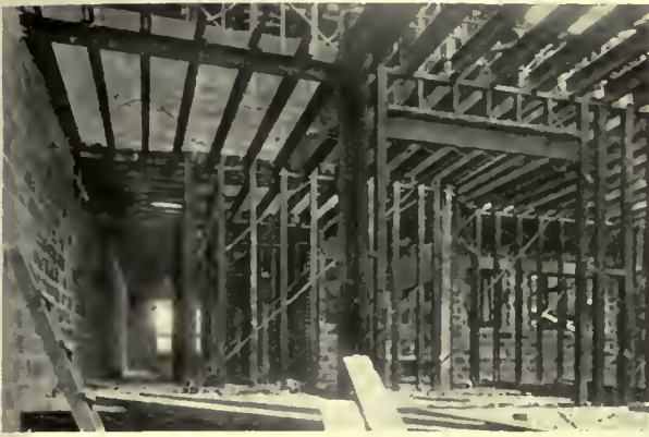
Apartment houses, Brookline, Mass., showing steel stud construction in all partitions, and steel joist floors
