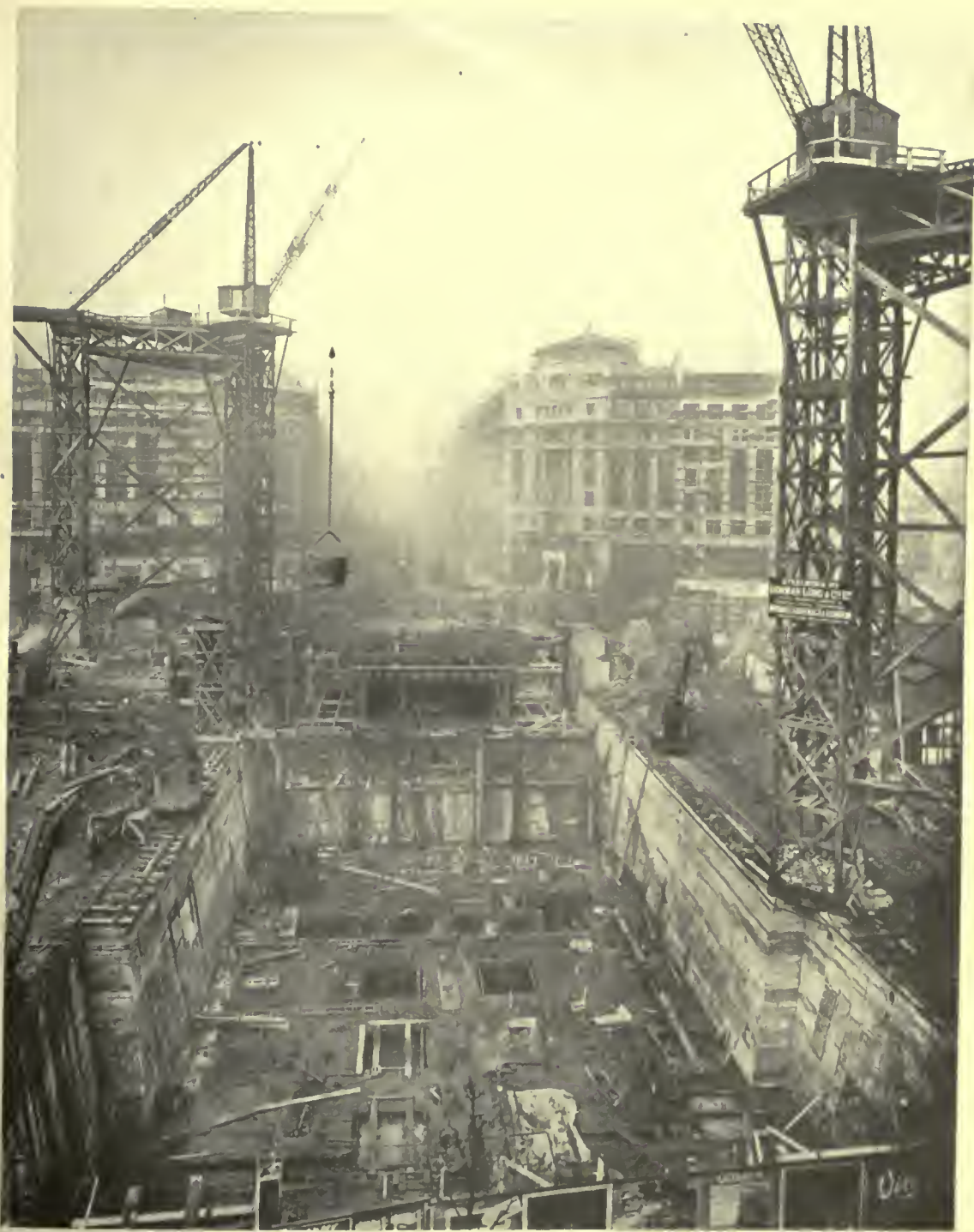
RETAINING WALLS COMPLETED AND COLUMN FOOTINGS UNDER WAY BUSH BUILDINGS, LONDON HELMLE & CORBETT, ARCHITECTS
