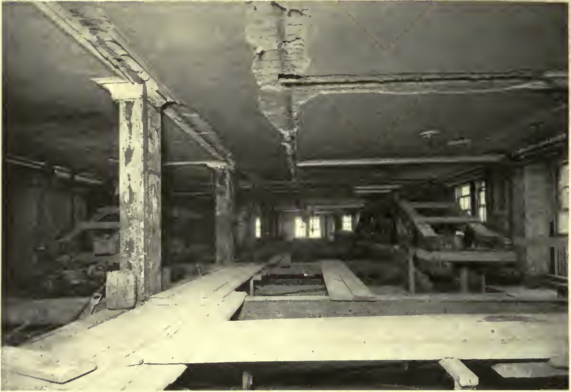
Heavy Trusses used to carry the girders which were hoisted into place by means of chain blocks. The cast iron columns here shown remain in the remodeled structure resting on girders
