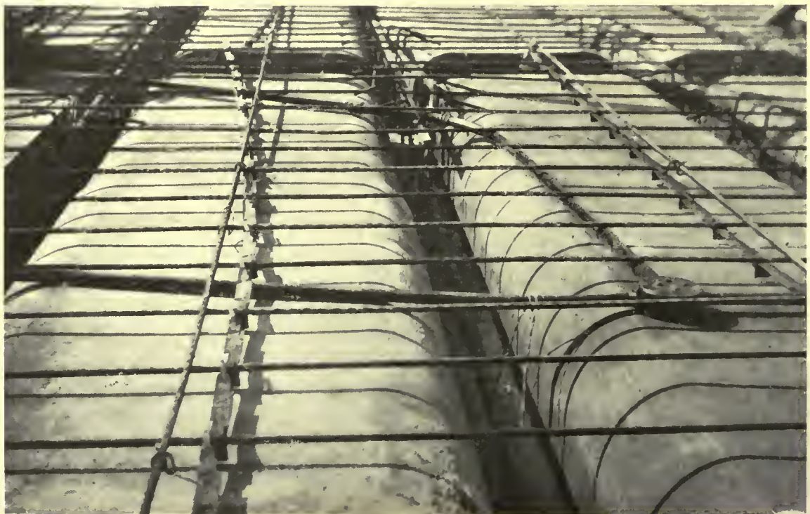
Metal centers in place for floor of Otis Building. Reinforcement supported on metal spacers to insure depth and spacing. Conduits for electric wires are embedded in the slab
