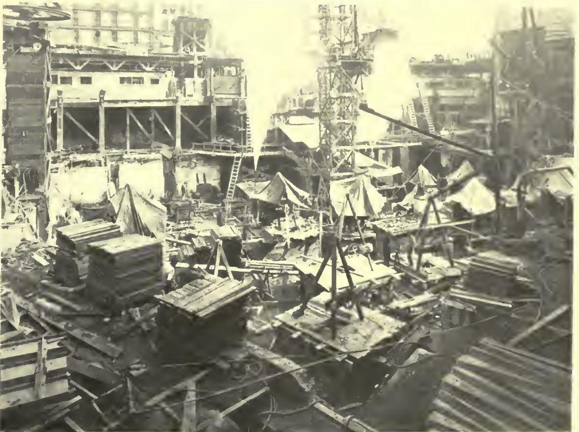
CONCRETING THE CAISSONS FOR BANK AND OFFICE BUILDING ON THE SITE OF THE OLD HOTEL PONTCHARTRAIN, DETROIT
