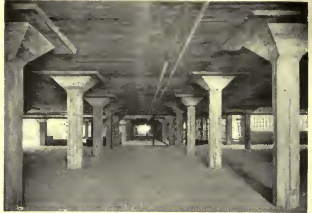
Reinforced concrete. Girderless floor carried on drop-heads supported by large column capitals. The columns are octagon in shape to harmonize with the square capitals and at same time resist fire practically as well as round columns.
