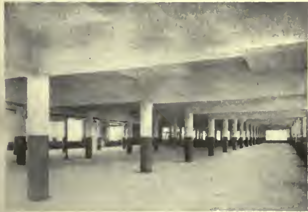
Reinforced concrete. Special design with deep, narrow girders carrying wide, shallow beams. Round columns.
