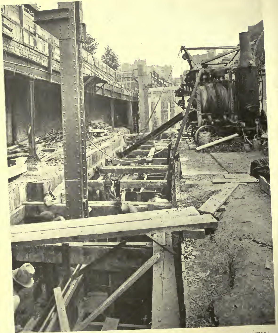
DETAIL VIEW OF EXCAVATION METHODS USED FOR END WALLS OF BASEMENT BUSH BUILDINGS, LONDON. HELMLE & CORBETT, ARCHITECTS
