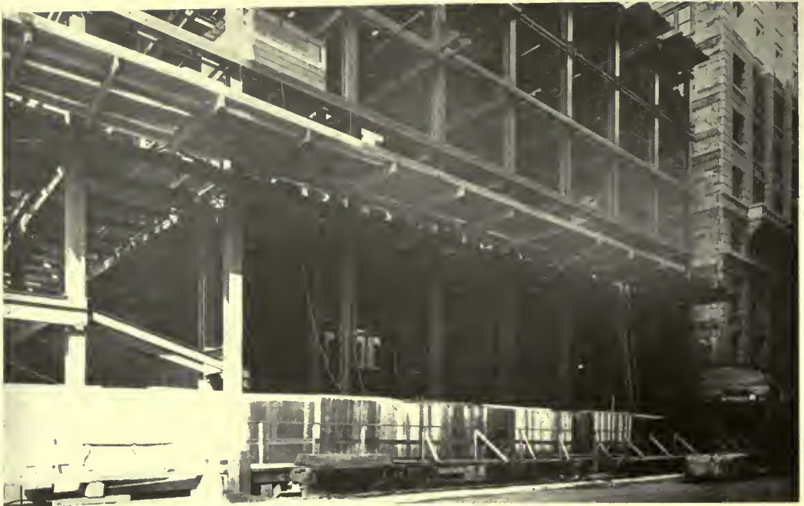
PROGRESS VIEW. SLOPING STEEL WORK FOR BALCONY CAN BE SEEN AT THE LEFT
