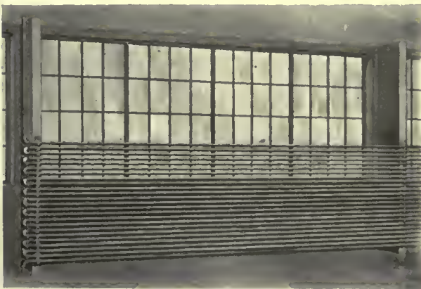
AN OBJECTIONABLE INSTALLATION
