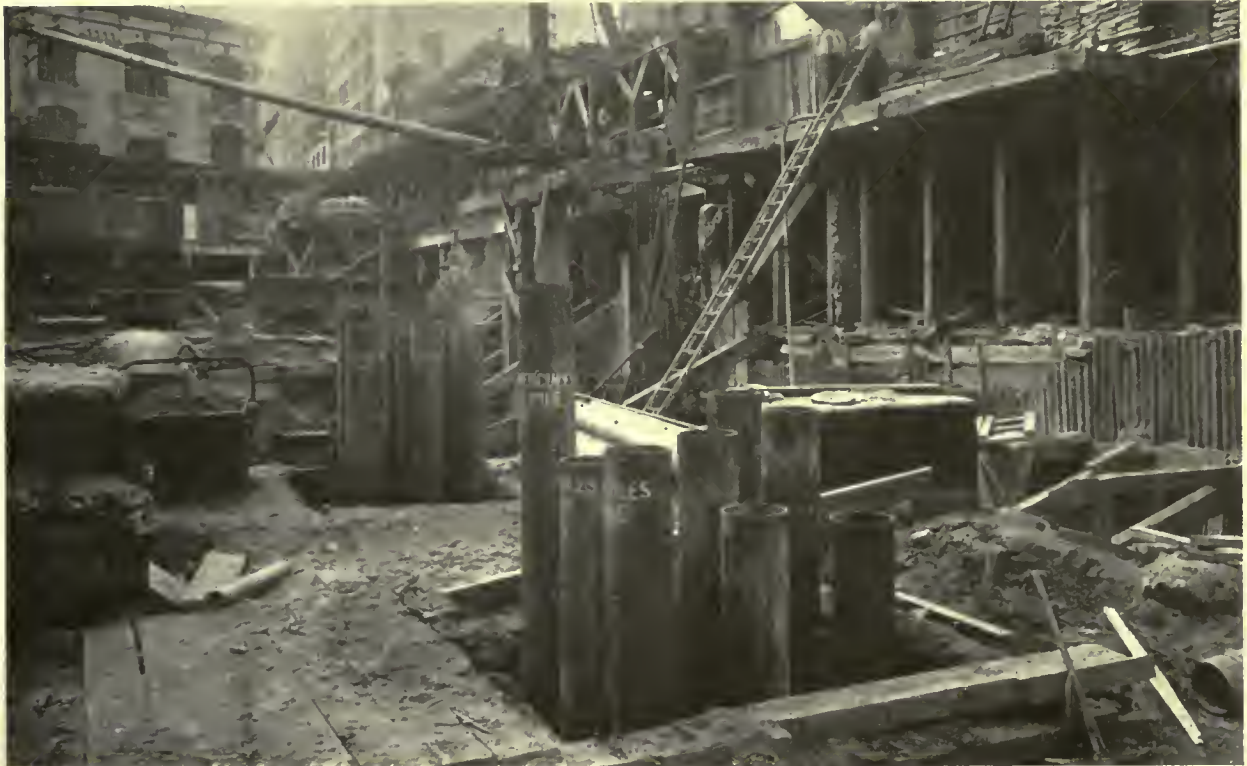
A FOUNDATION IN WHICH HERCULES TUBULAR PILES, DRIVEN TO ROCK, WERE USED That part of the steel tube which projects above the specified level is cut off by the use of the oxy-acetylene burner
