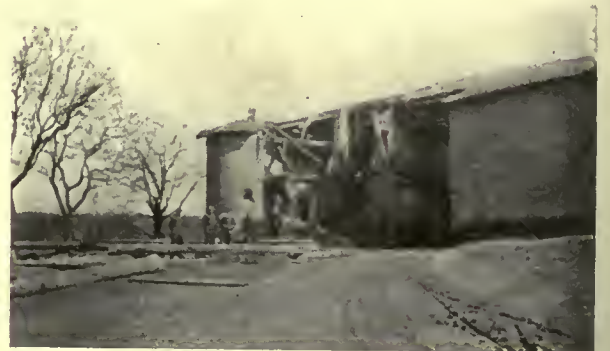
THE VISIT OF A BOMB REVEALS OLD METHOD OF CONSTRUCTION
