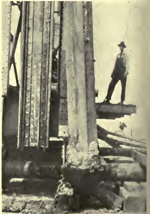
CLOSE UP VIEW, SHOWING CONDITION OF C. I. DRIVING POINT AND CONCRETE
