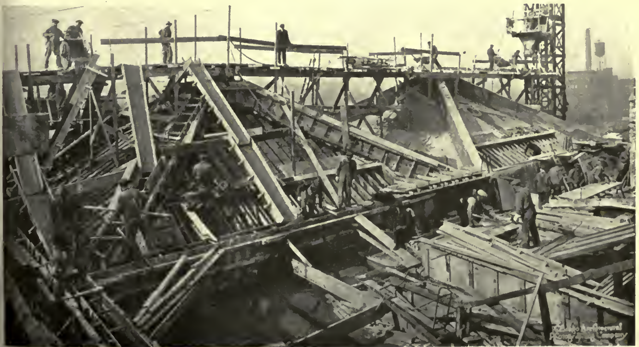
UNUSUAL ROOF CONSTRUCTION—NOTE REINFORCED CONCRETE HIP GIRDERS N. MAX DUNNING, ARCHITECT. LIEBERMAN, KLEIN & HEIN, ENGINEERS
