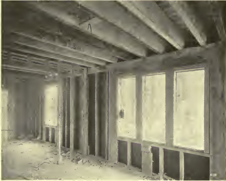
FIG. 3. INSIDE VIEW OF WALL, SHOWING CONCRETE STUDS, ALSO SPECIAL LINTEL OVER TRIPLE WINDOW
