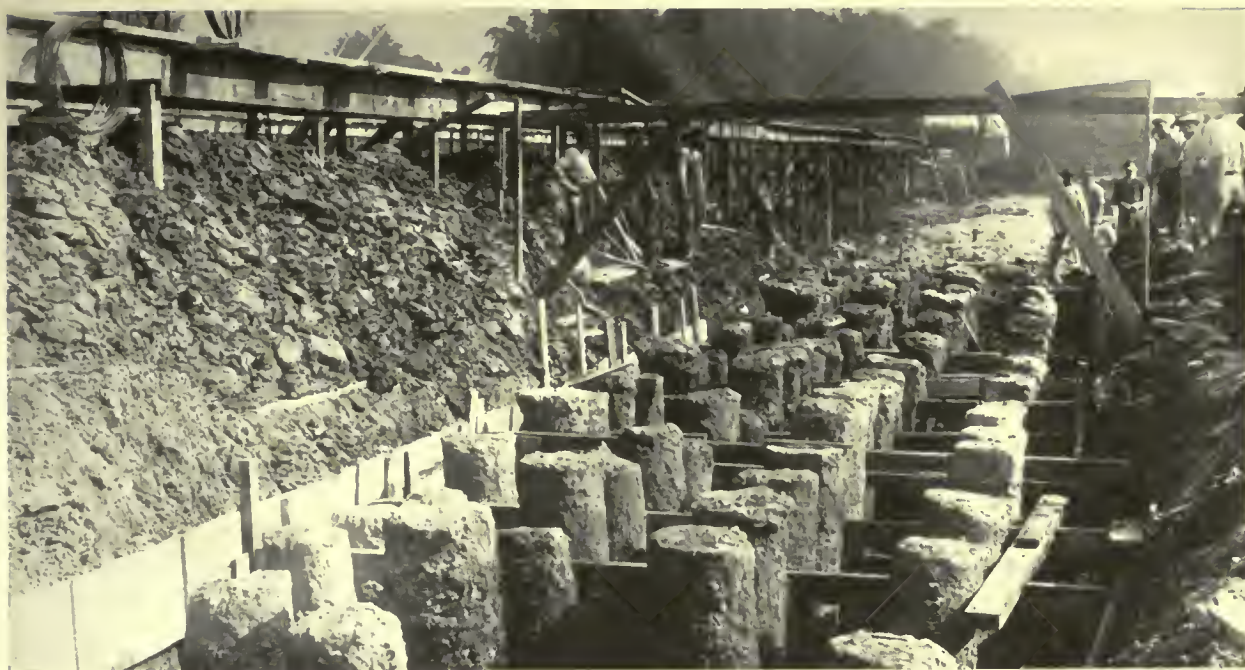
GROUP OF PEDESTAL PILES FOR THE WILLYS-OVERLAND COMPANY'S PLANT AT TOLEDO, OHIO Earth around tops of piles excavated and forms being placed for concrete cap
