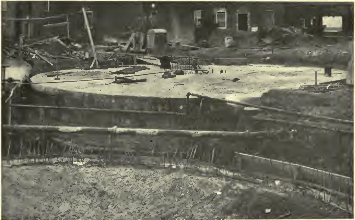
VIEW SHOWING ONE COMPLETED TANK AND ANOTHER UNDER CONSTRUCTION BOSTON RUBBER SHOE CO., PLANT NO. 1, MALDEN, MASS.
