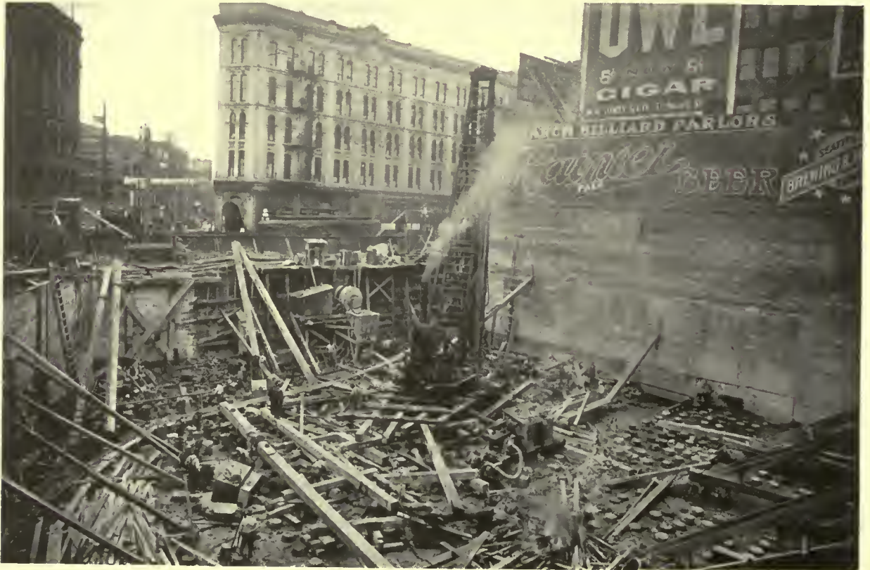
PILE DRIVING IN PROGRESS FOR THE L. C. SMITH BUILDING, SEATTLE, WASH.
