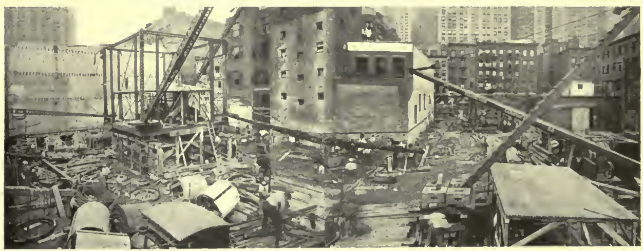
COMMENCEMENT OF FOUNDATION WORK ON THE BARRETT BUILDING, NEW YORK CITY Note cutting edges with vertical reinforcement (at left) in place for circular caisson construction
