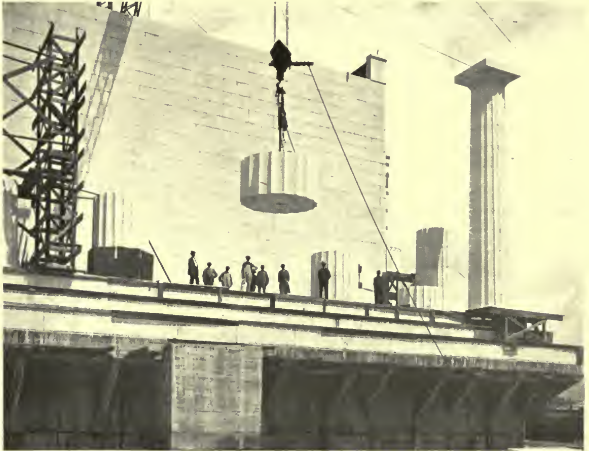
PLACING THE COLONNADE THE LINCOLN MEMORIAL, WASHINGTON, D. C. HENRY BACON, ARCHITECT
