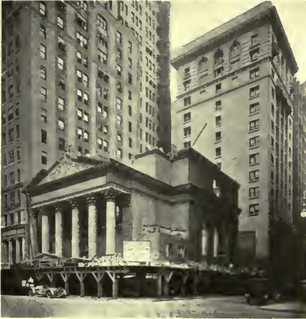
SITE OF THE NEW METROPOLITAN ANNEX Demolition of Madison Ave. Presbyterian Church in progress.
