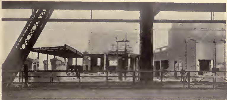
VIEW OF MAIN ROOF FORMING ENTRANCE TO STOREHOUSE BUILDING FROM BRIDGE. PASSENGER ELEVATOR BULKHEAD AND GARAGE TO RIGHT. FREIGHT ELEVATOR BULKHEAD TO THE REAR
