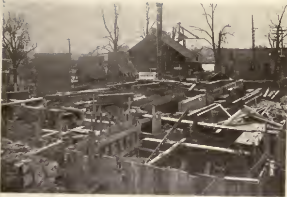
NO. 1. FOUNDATION WORK IN PROGRESS. SOME OF C. I. COL. BASES SET; PART OF STEEL ON JOB AND READY FOR ERECTION. BUILDING OF BRICK WALLS COMMENCED
