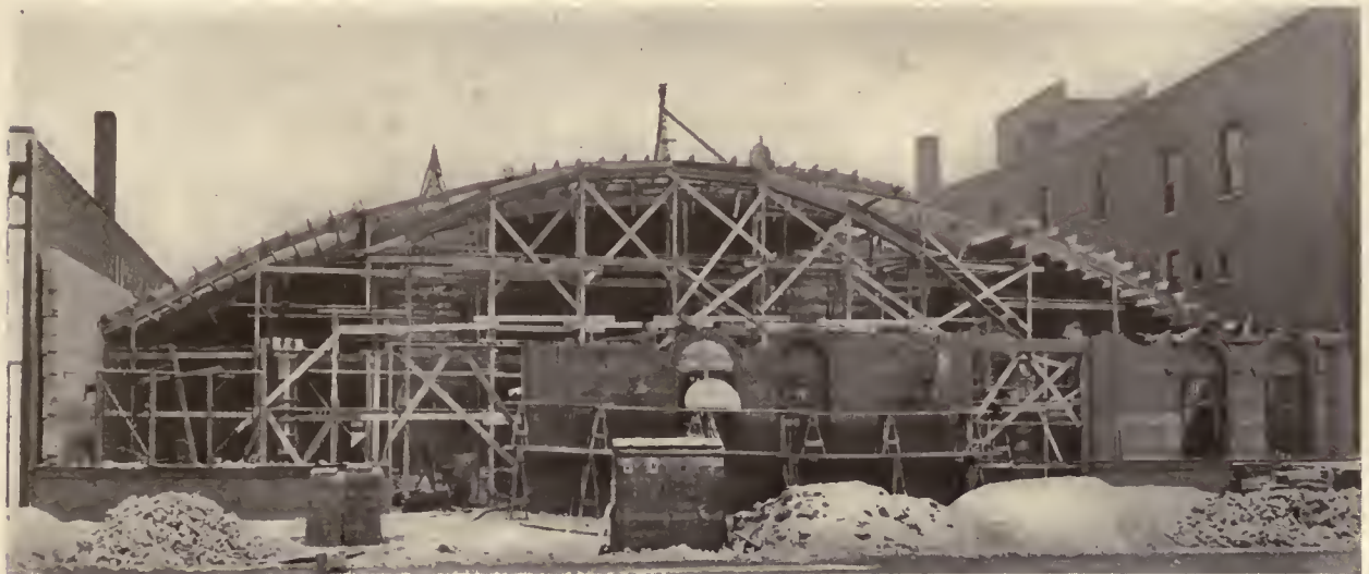
COTTAGE GROVE AVENUE END OF GARAGE DURING CONSTRUCTION. NOTE FALSEWORK SUPPORTING FORMS FOR CONCRETE ROOF ARCHES
