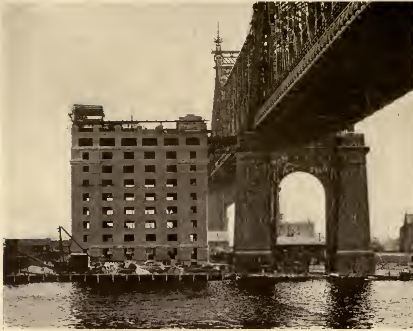
THE STOREHOUSE BUILDING NEARING COMPLETION. SUBWAY TUNNEL RUNS DIRECTLY UNDERNEATH BUILDING AND 125 FEET BELOW LEVEL OF BASEMENT FLOOR. OPERATION OF THIS SUBWAY IS SCHEDULED TO START APRIL 1
