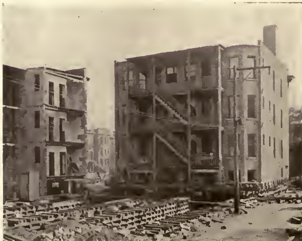
REAR OF SECTION 1 LOOKING EAST. THE BUILDING IS MOVED INTO IRVING AVENUE AND READY TO BE TURNED 180 DEG. ON ITS CENTER. TO THE LEFT IS REAR OF SECTION 2. NOTE THE SILLS, ROLLERS AND CRIBBING.
