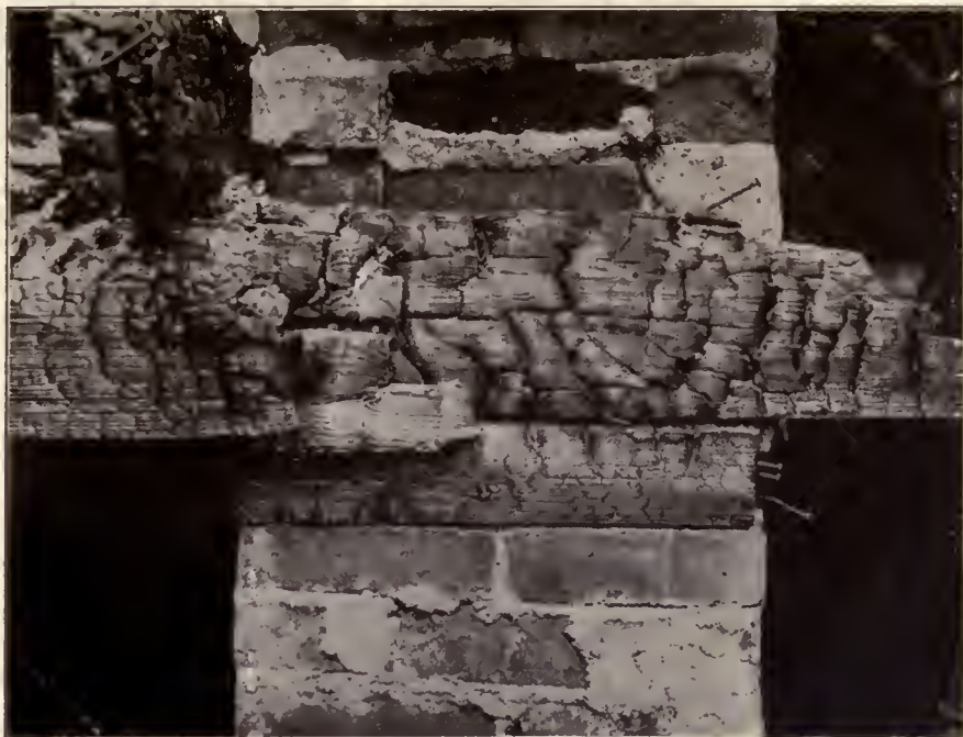
RESULT OF POOR CHIMNEY CONSTRUCTION. FLOOR ATTACHED TO CHIMNEY HAVING ONLY 4-INCH WALLS AND NO LINING. FIRE DESTROYED BUILDING
