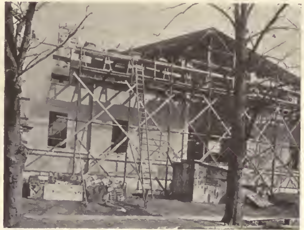
NO. 4. THREE MONTHS LATER. FLOOR AND ROOF ARCHES COMPLETED. WALLS NEARLY TOPPED OUT
