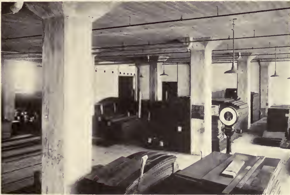
THE OAKES COMPANY BUILDING, INDIANAPOLIS VONNEGUT, BOHN & MUELLER, ARCHITECTS. INTERIOR VIEW SHOWING THE TEMPORARY DRAINS FROM THE ROOF.
