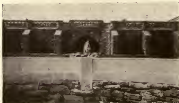
COPING OF CIRCULAR WATER BASIN AND BALUSTRADE OF CAST STONE; WALLS OF LOCAL QUARRY STONE. ROSEMONT, PENNA.
