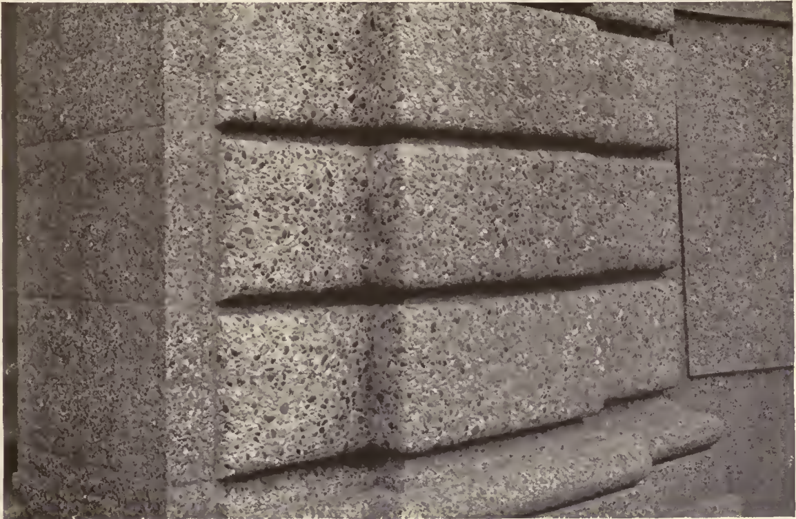
FIG. 5. DETAIL VIEW OF ENTRANCE TO MERIDIAN HILL PARK, WASHINGTON, D. C., SHOWING EXPOSED AGGREGATE SURFACES
