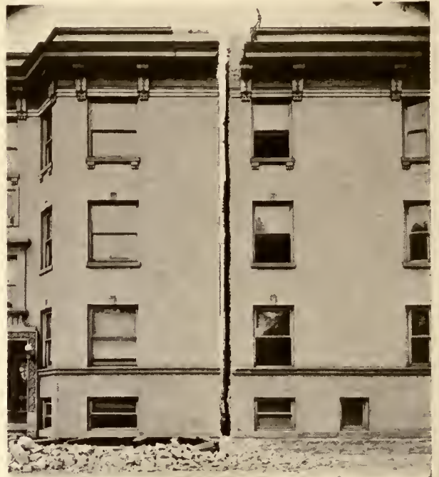
CUTTING THE BUILDING INTO TWO SECTIONS, SECTION 1 AT LEFT AND SECTION 2 AT RIGHT. SECTION 1 "LOADED" ON THE FALSEWORK READY TO BE RAISED PREPARATORY TO MOVING.
