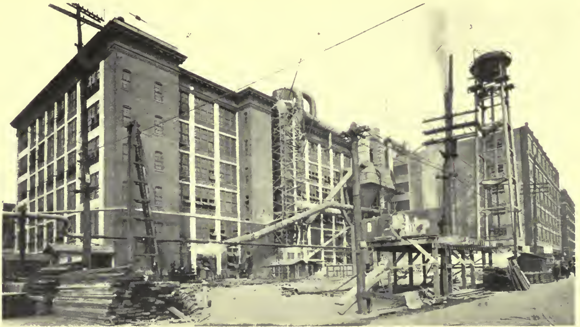
Site of Building 17D, with Buildings 17, 17A at left and center with 17C back of water tower. Building No. 1 at extreme right. Old water tower being wrecked. Note elevated steam main entering at the left and later placed in tunnel.
