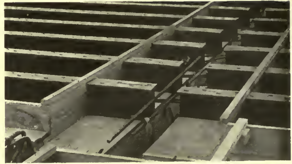
Reinforced concrete T-beam girder with metal floor joists in place and anchored together, ready to be poured.
