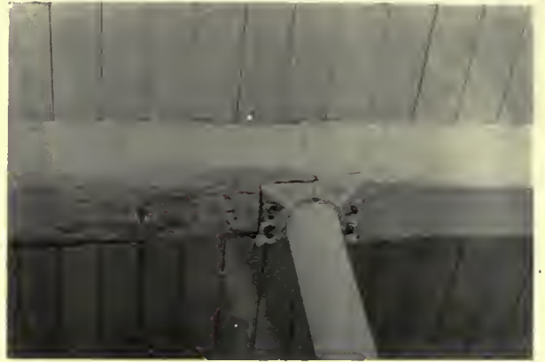
Fig. 18. Cast iron columns used as a drain pipe for rain water has precipitated water on and seriously rotted the beams which enclose it.
