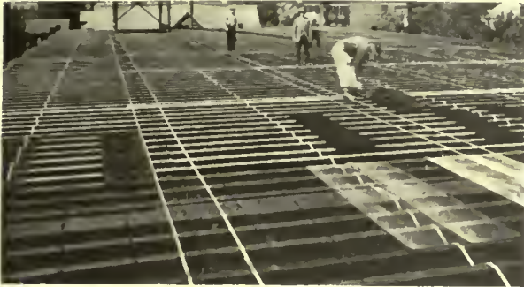
Placing the metal lath over metal floor joists. The white strips are galvanized iron bands used as bridging to keep the joists in position until the concrete slab is placed.
