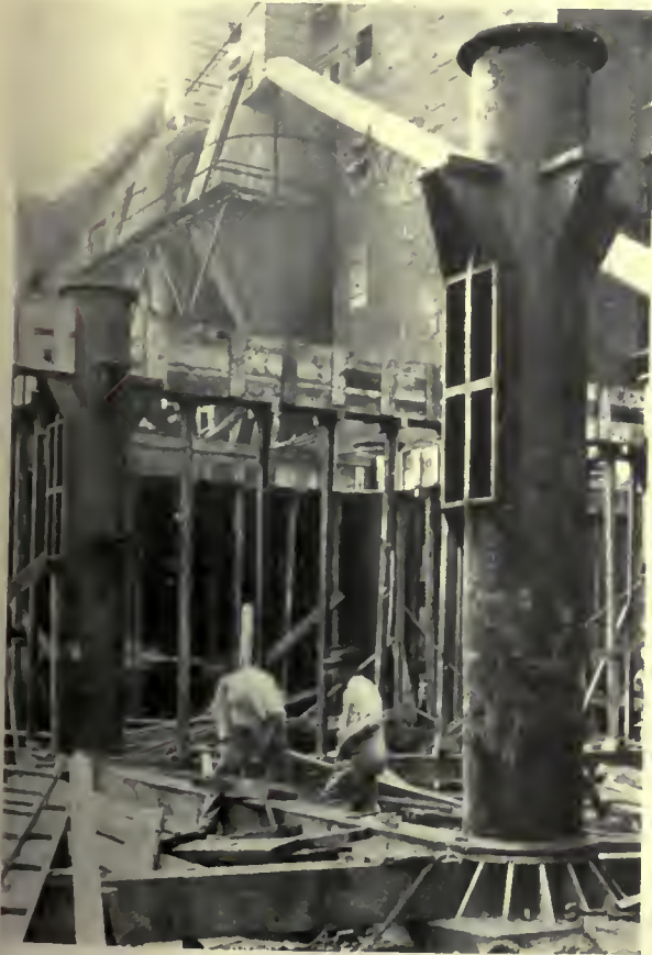
Basement column in position, showing brackets for supporting the floor slab and openings for hot air registers
