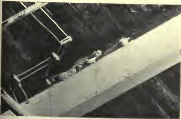
Fig. 6. Fomes Officinalis plants growing on the side of a beam under a weave-shed roof from which the sheathing has been removed for some time.
