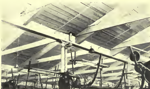
Fig. 17. This iron pipe, for carrying away rain water from the roof, has absorbed sufficient heat to precipitate water on the nearby roof, causing the roof to rot.
