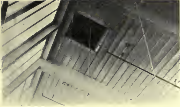
Fig. 20. Roof rotted for 10 or 15 feet from a ventilator, owing to the escape of heat, reducing the temperature and causing moisture to precipitate on the roof planks.
