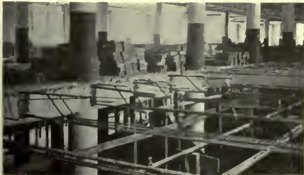
Condition of outer bay after concrete had been removed. Note beam reinforcing rods left in place; also that cases of sheet tin stacked in center penal are located over girders.
