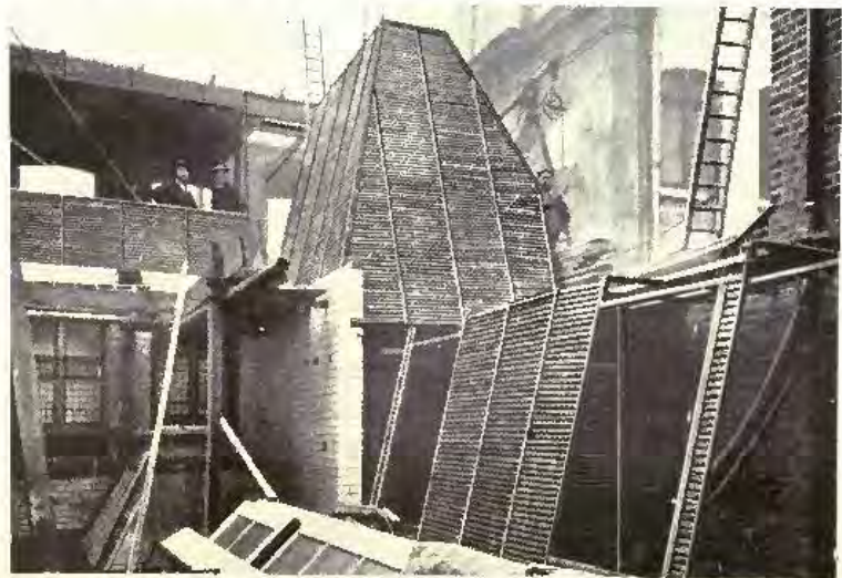
PHOTO OF ROOF WORK IN DOVETAIL CORRUGATED STEEL SHEETING. SUPPLIED AND FIXED BY THE FIREPROOF CO., LTD.
