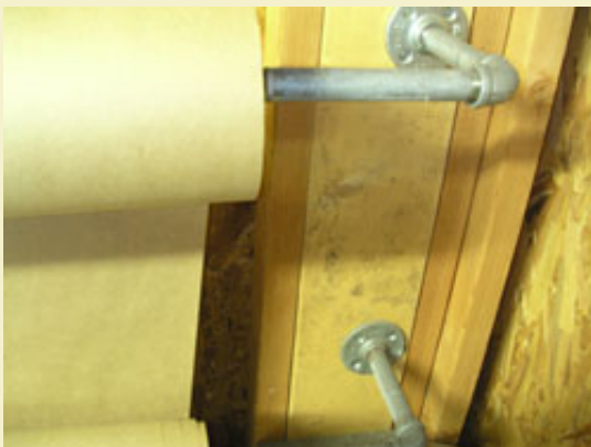
Figure 3: Pipe fittings used to hang paper rolls.
