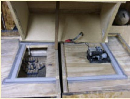
Figure 9: Underneath the air hood on top.
