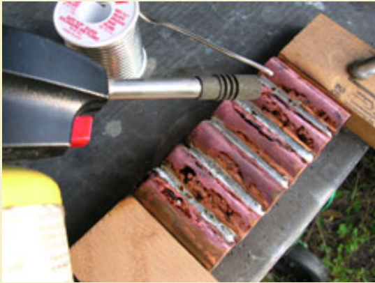
Figure 3: Using a blowtorch to run a bead of solder between each pipe.
