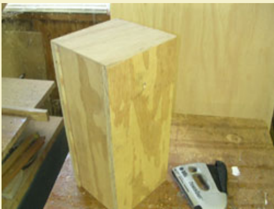
Figure 3: After the box is glued together, the bottom is closed with a scrap of thin wood to hold in the wet concrete when the box is filled.
