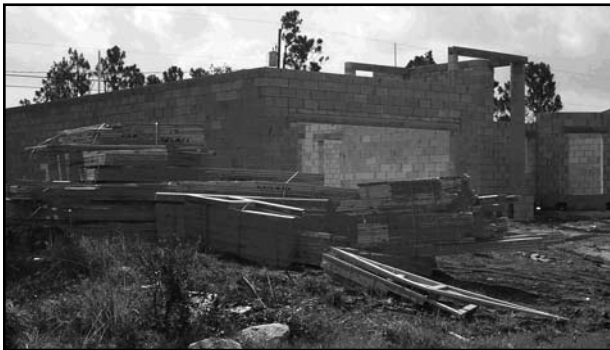
Example of large scale building materials being left unprotected during the early stages of a construction site.
