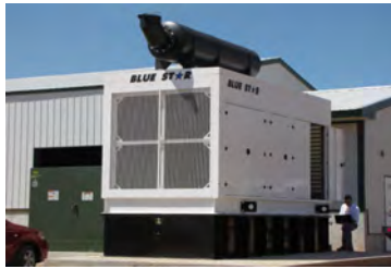
Typical external appearance of a transportable diesel generator set.
