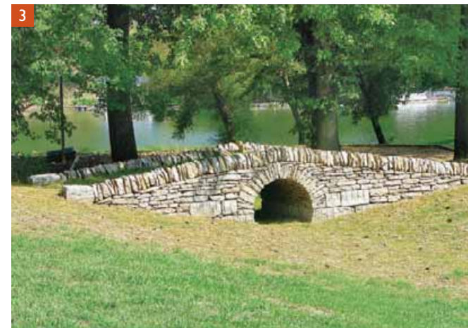
[1] Low dry-stone walls coupled with pavers laid without grout (an offshoot of walling) create a terrace that looks centuries old. [2] Waller James Asbury reconstructed this 100-year-old Mansfield, Pennsylvania, retaining wall breached by a nearby tree. If not for the encroaching roots, the interlocking flagstone would have stood sentry over the hillside for years. [3] This dry-laid sandstone arch bridge in Frankfort, Kentucky, spans a low-lying area without impeding water flow.
