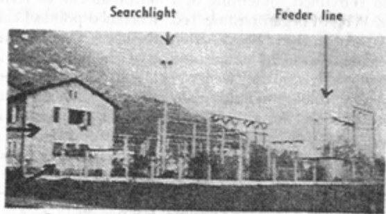
Overall view of a transformer station
